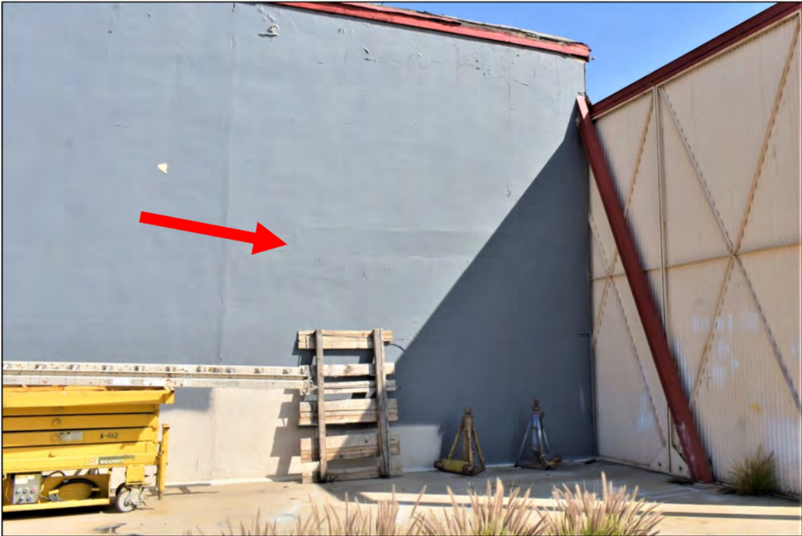
Figure 46: Building 7 South elevation showing an early patch to the original stucco.
