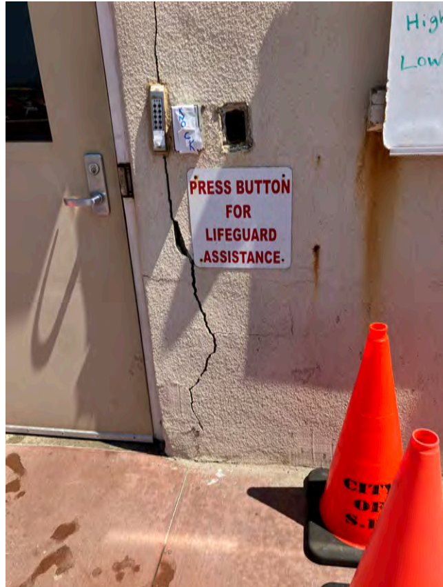
PHOTO 4: CRACKS AT ENTRY DOOR ON WEST SIDE
