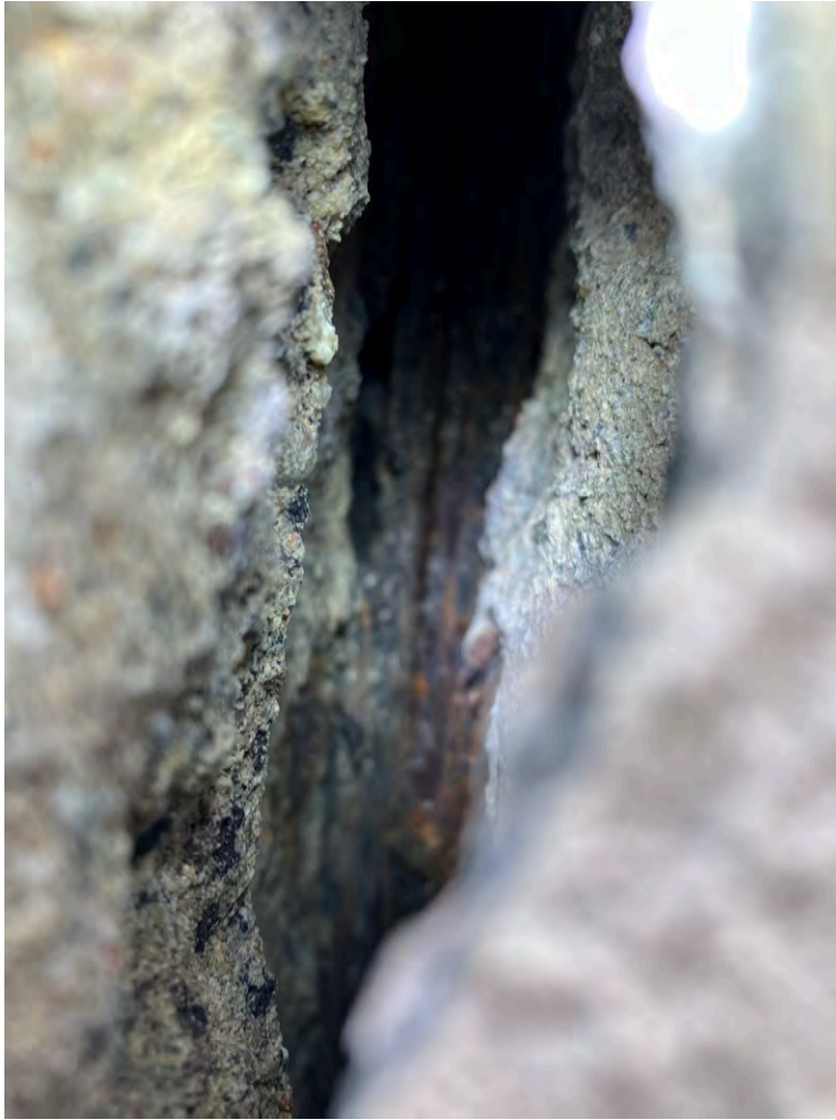
PHOTO 7: CLOSEUP OF REINFORCING STEEL AT CRACK AT SOUTHWEST CORNER
