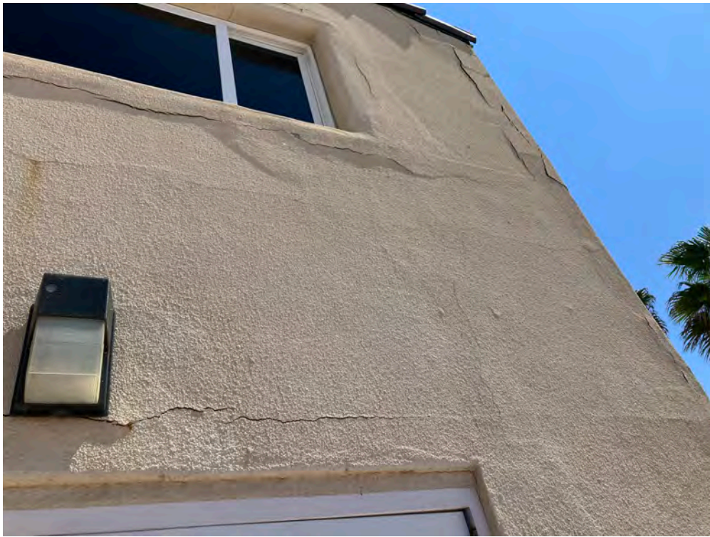
PHOTO 5: CRACKS AND DELAMINATION AT SOUTH END OF WEST SIDE
