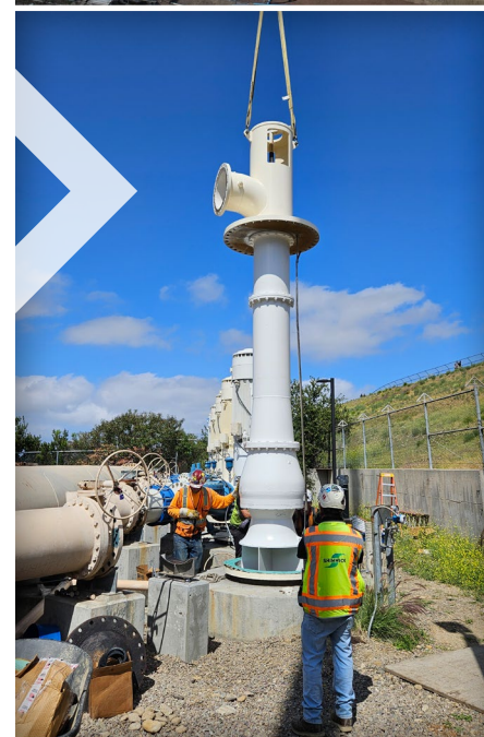
Miramar Reservoir Pump Station
