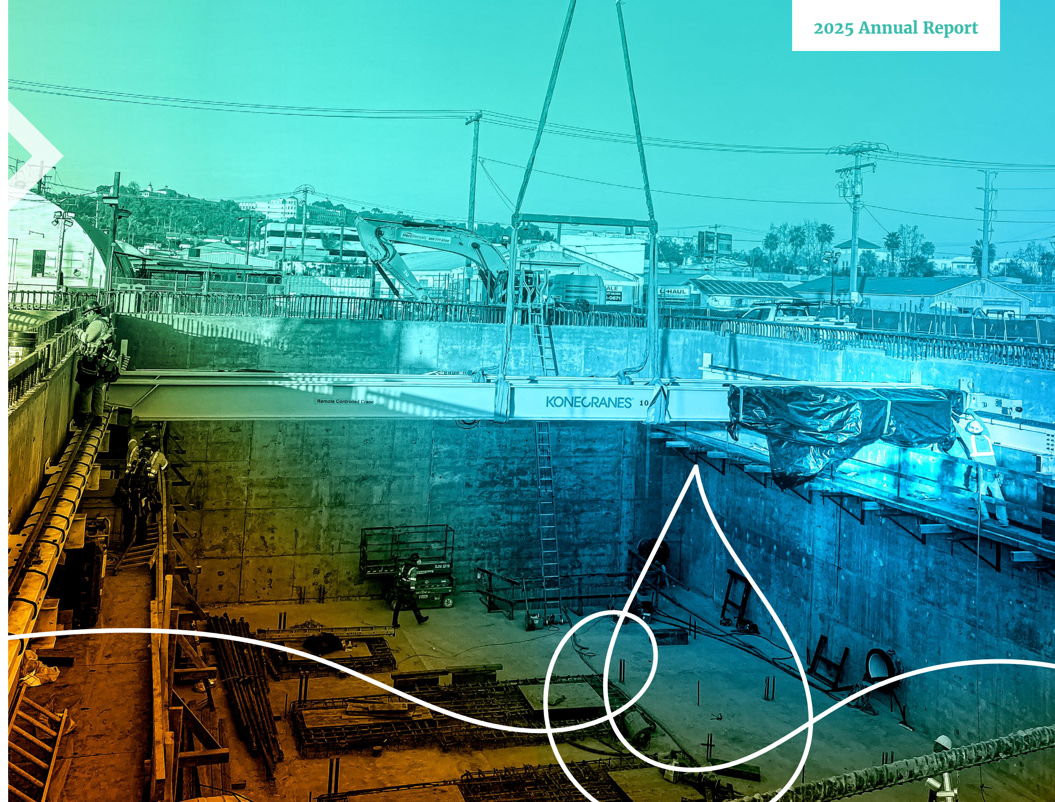
Morena Pump Station
