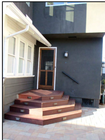
2021 View from the Southeast Corner showing the vertical hyphen connection from the historic residence to the addition, Landmark Historic Preservation , pg. 105
