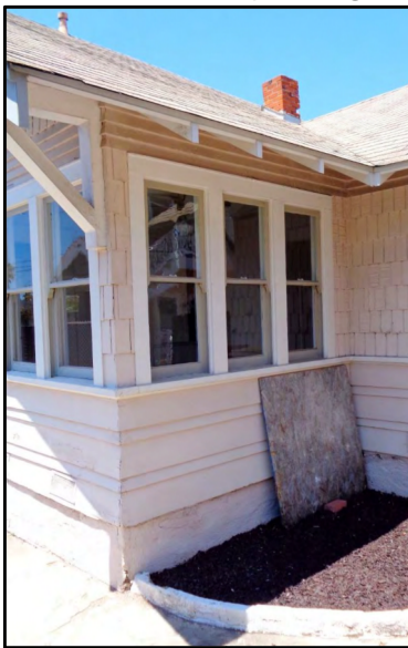
2020 View from the Southeast Corner showing pre-project east-facing open eave ends, Landmark Historic Preservation, pg. 87
