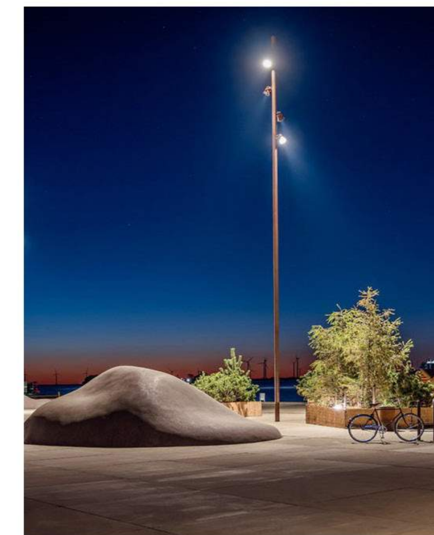
★ Area Pole Lighting 18'
