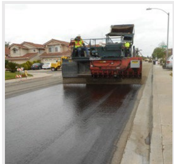
Slurry seal is applied after the crushed rock layer has cured for 3 days
