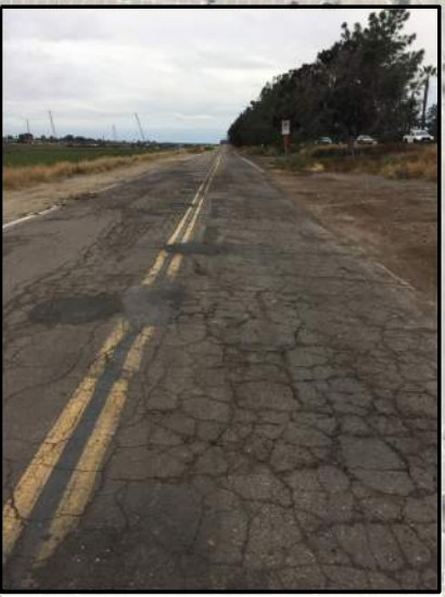
4 UNEVEN PAVEMENT WITH NUMEROUS POTHOLES (LOOKING WEST)
