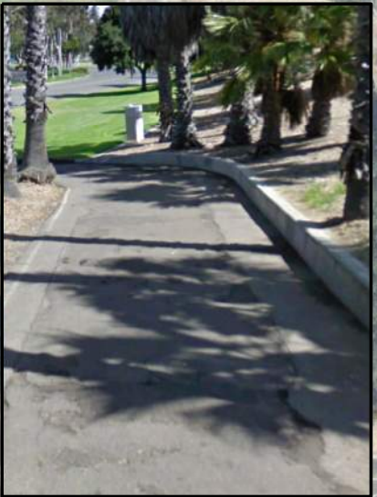
3 4 POOR PAVEMENT CONDITION (LOOKING NORTH)
