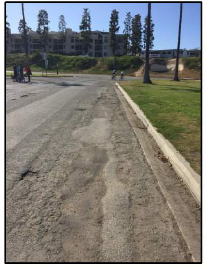
2 PAVEMENT IN POOR CONDITION (LOOKING WEST)
