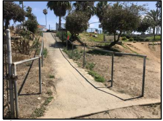
2 EXISTING RAMP FOR PEDESTRIANS AND CYCLISTS IS NOT ADA COMPLIANT AND POSES SAFETY CONCERN (LOOKING SOUTH)
