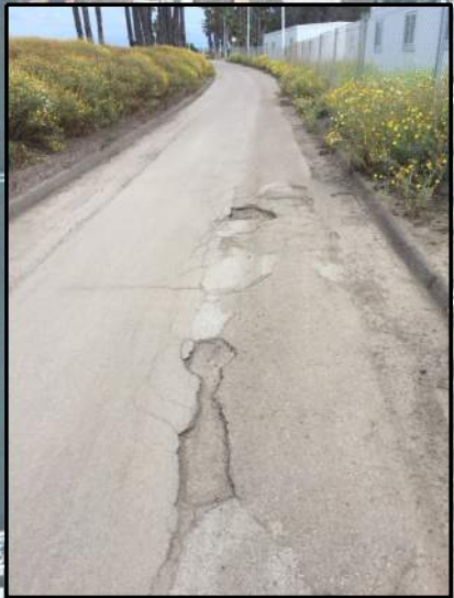
2 POOR PAVEMENT CONDITION (LOOKING WEST)
