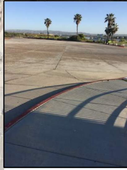
2 SHARED USE PATH ENDS, MISSING ADA CURB/BIKE RAMP TO EXIT FACILITY (LOOKING NORTH)
