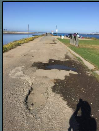
1 SHARED-USE PATH PAVEMENT IN POOR CONDITION (LOOKING WEST)
