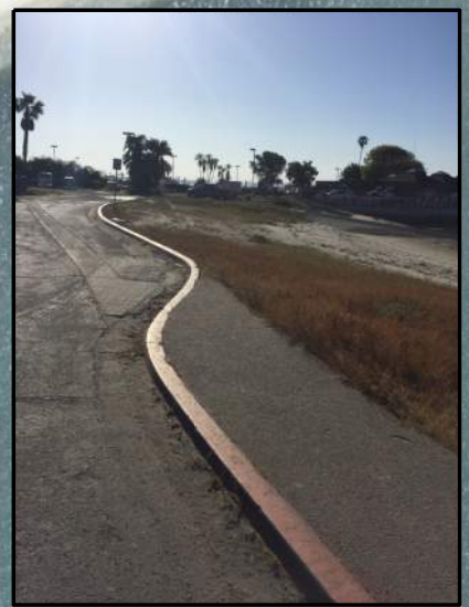
1 EXISTING PEDESTRIAN PATH DEAD ENDS (LOOKING EAST)
