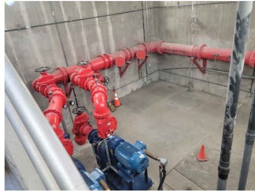
Recently Upgraded PS 23 with spare room for additional pumps.
