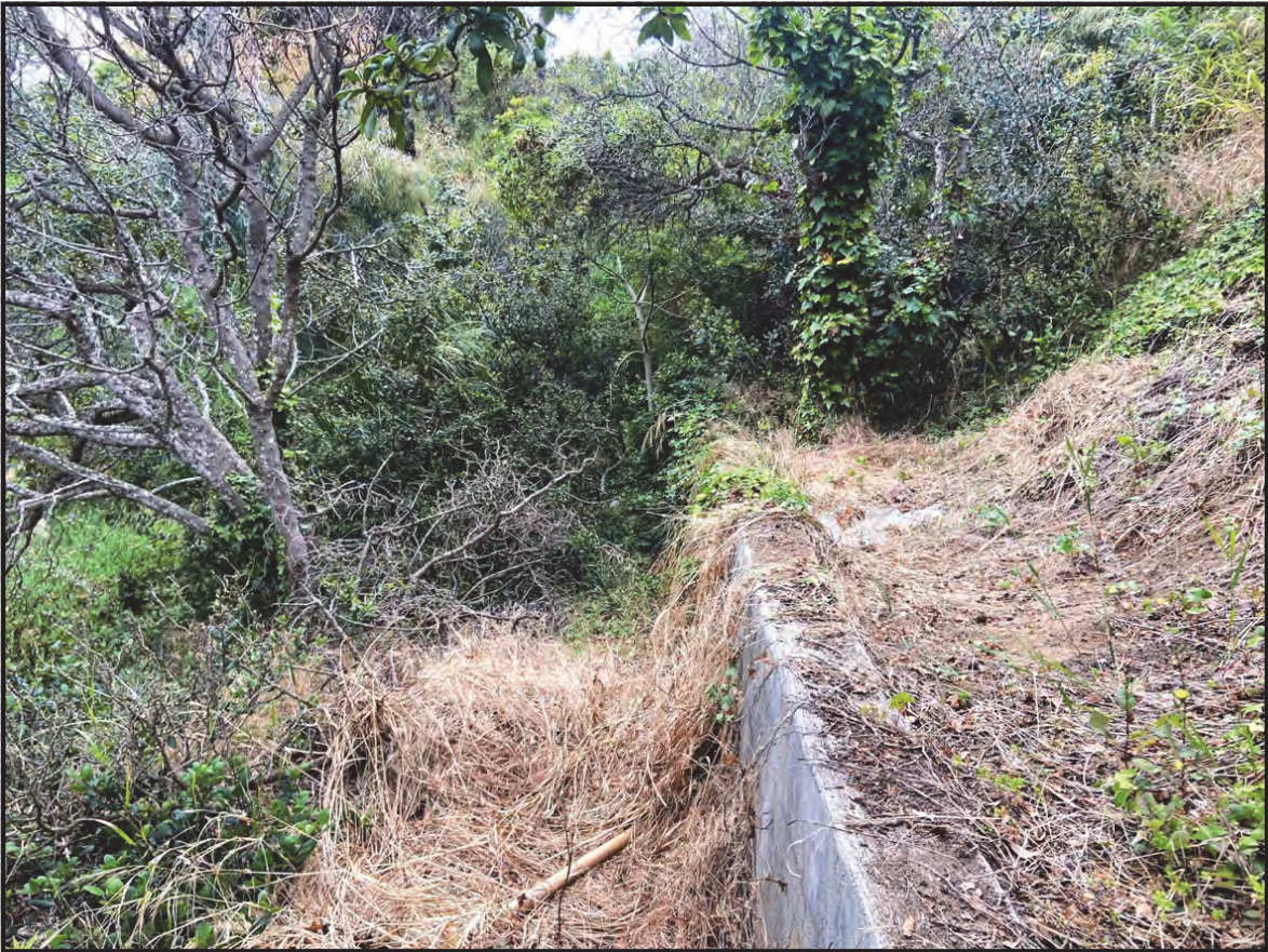
3. Retaining wall in the Developed area below the existing residence's lower terrace (from lower-central Developed toward north/northeast).
