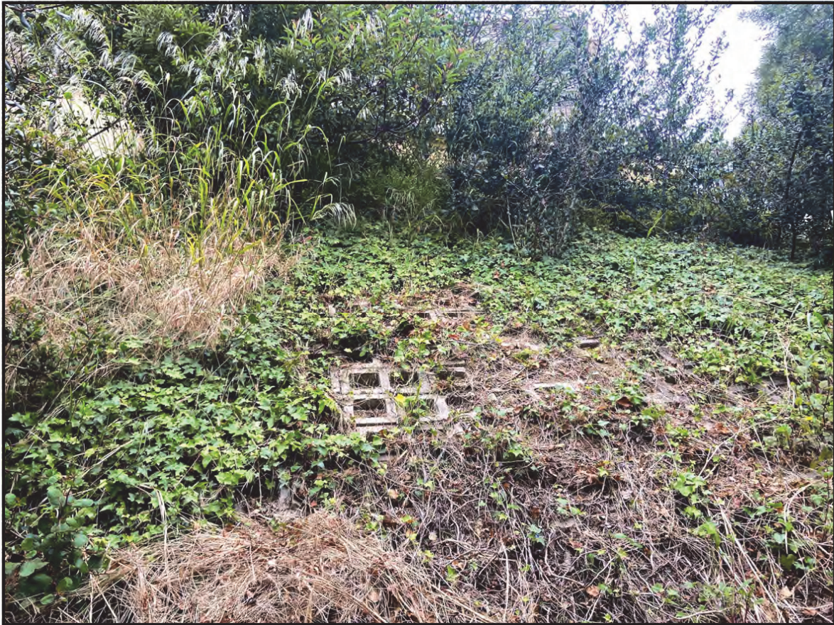
2. Concrete slope reinforcement on the Developed Land below the residence's lower terrace (from near southern boundary toward southeast).
