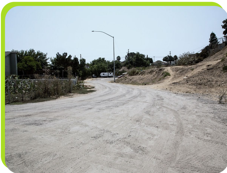
Example of an unimproved street requiring significant investment for full construction and drainage improvements.
