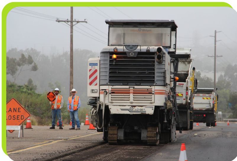
Traffic control in place to safely guide vehicles through active paving operations.
