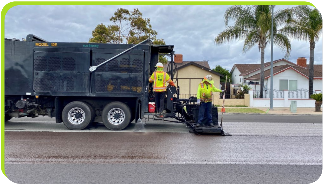
Contractor applying slurry seal to preserve pavement condition and extend the life of existing streets.
