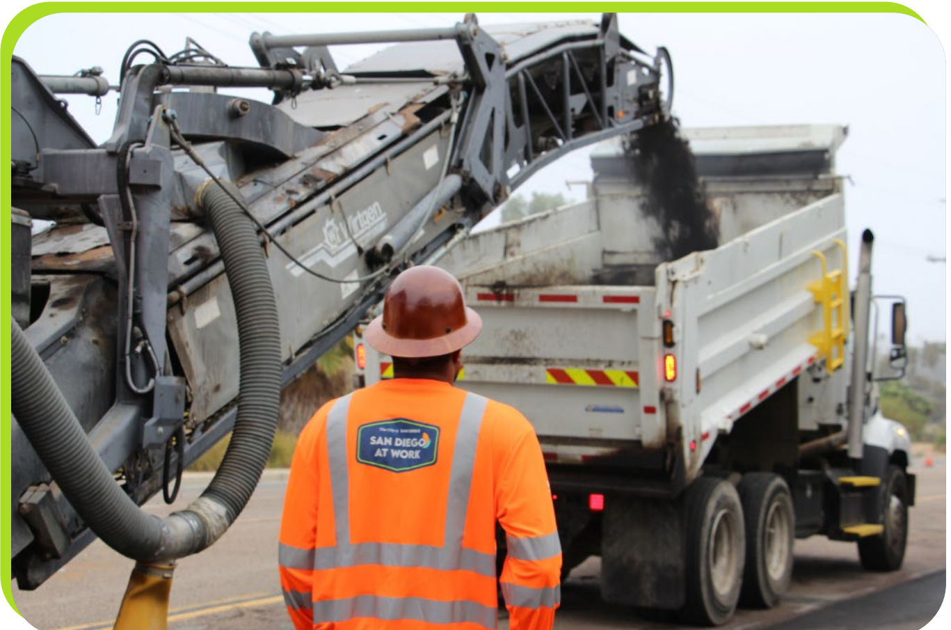
The City's milling machine removing existing asphalt and loading material for recycling during pavement rehabilitation.
