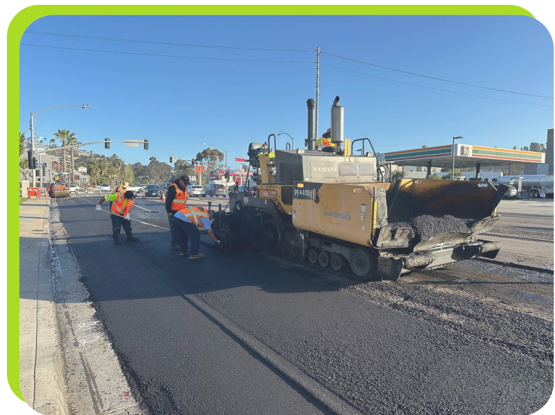
In-house paving crew placing new asphalt to restore roadway surface and extend pavement life.
