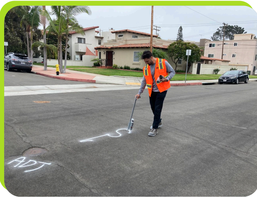
City engineering staff performing field mark-outs to support coordination and implementation of slurry seal projects.
