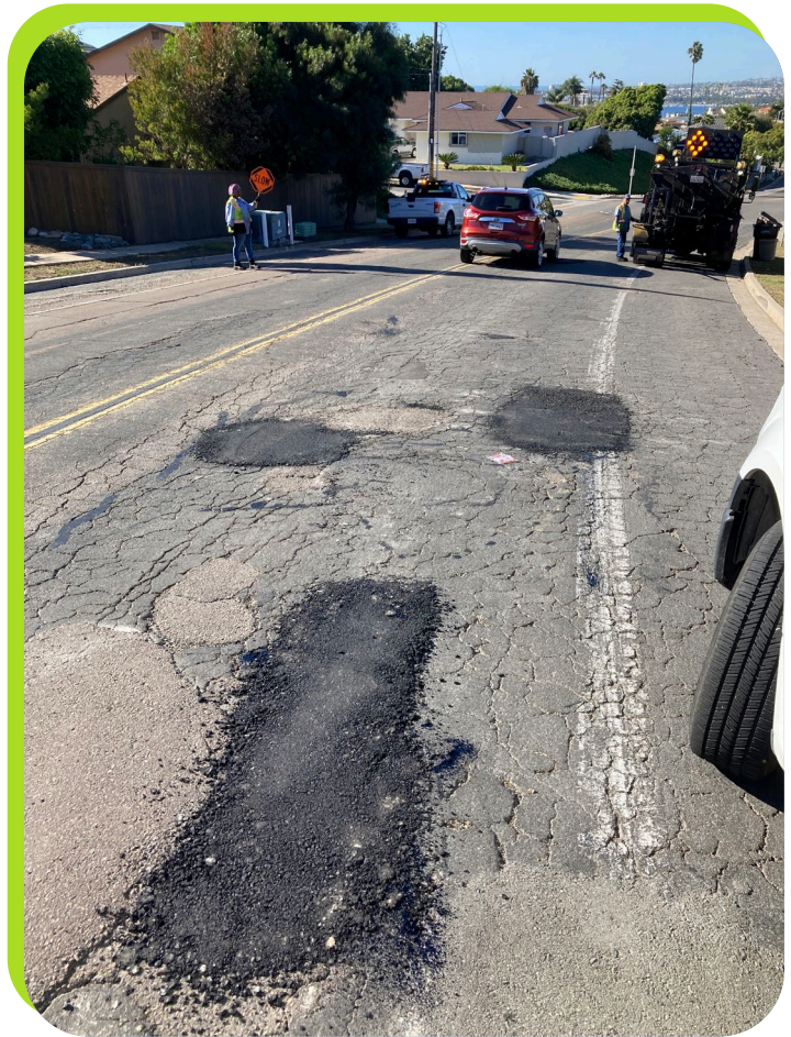
Example of deteriorated pavement conditions requiring more extensive rehabilitation as streets transition from fair to poor conditions.
