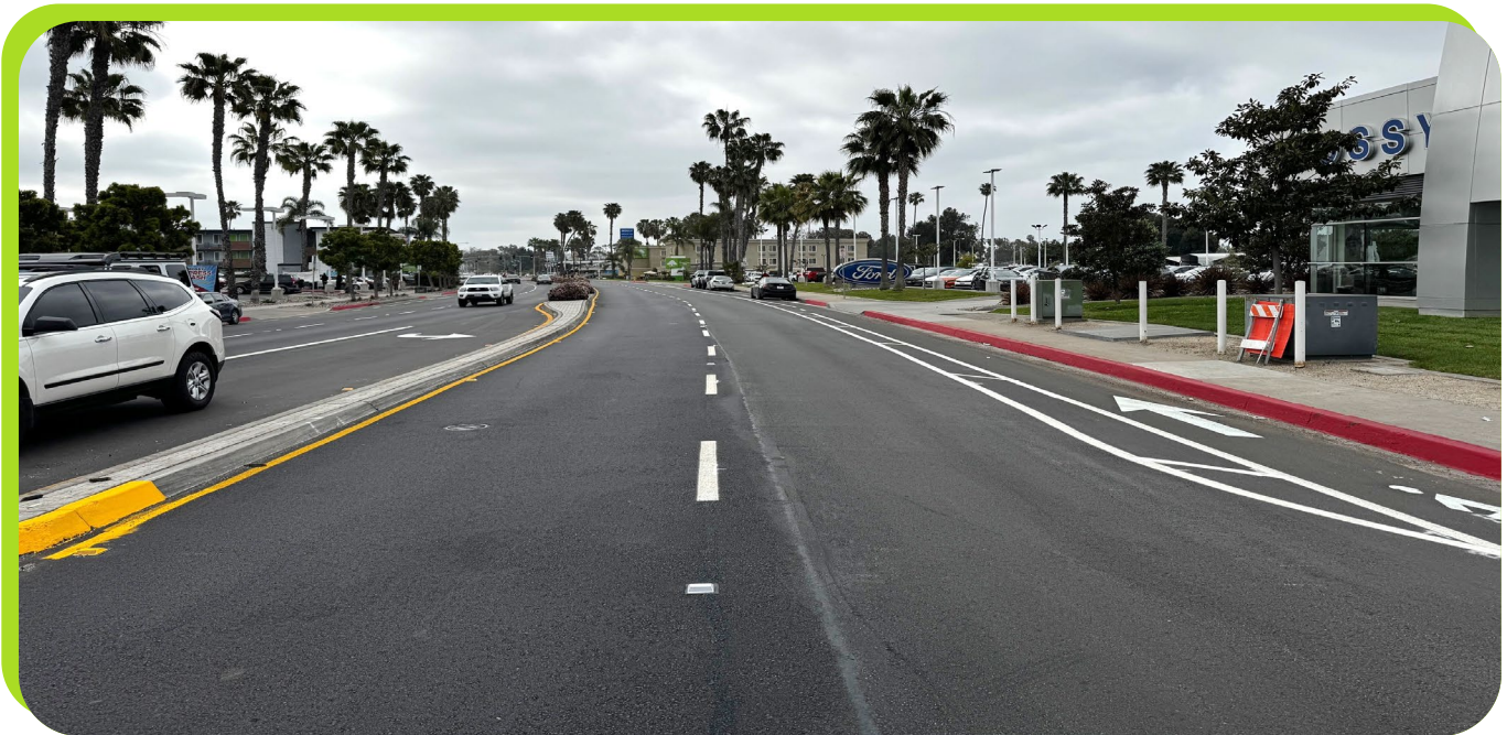
A photo of a recently paved Mission Bay Drive performed by the in-house Mill & Pave team.
