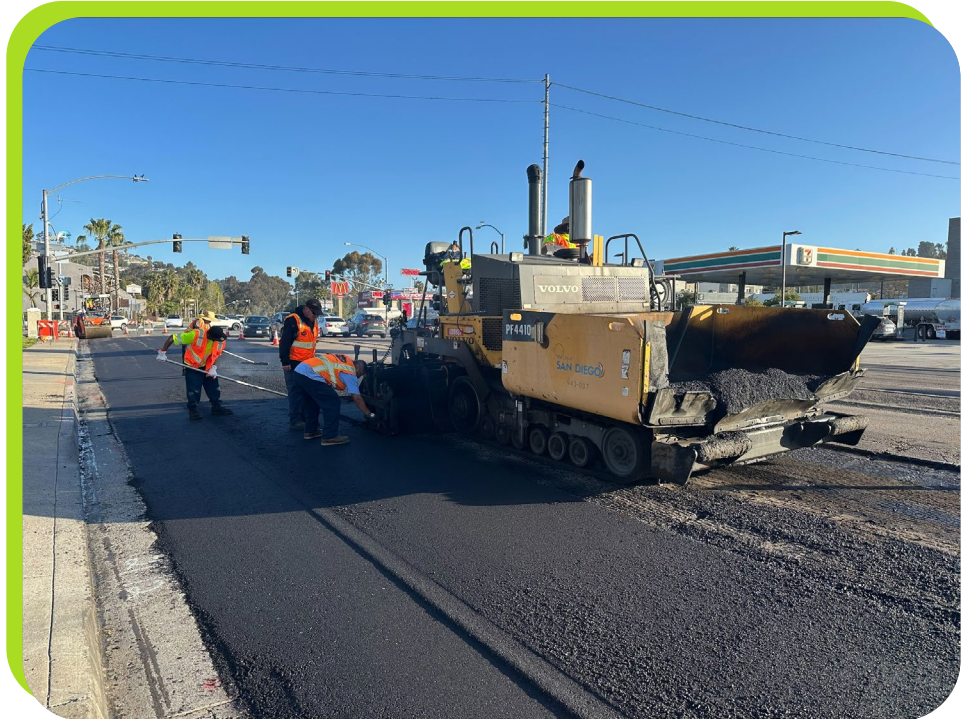
City in-house team performs asphalt placement to rehabilitate streets in poor condition.
