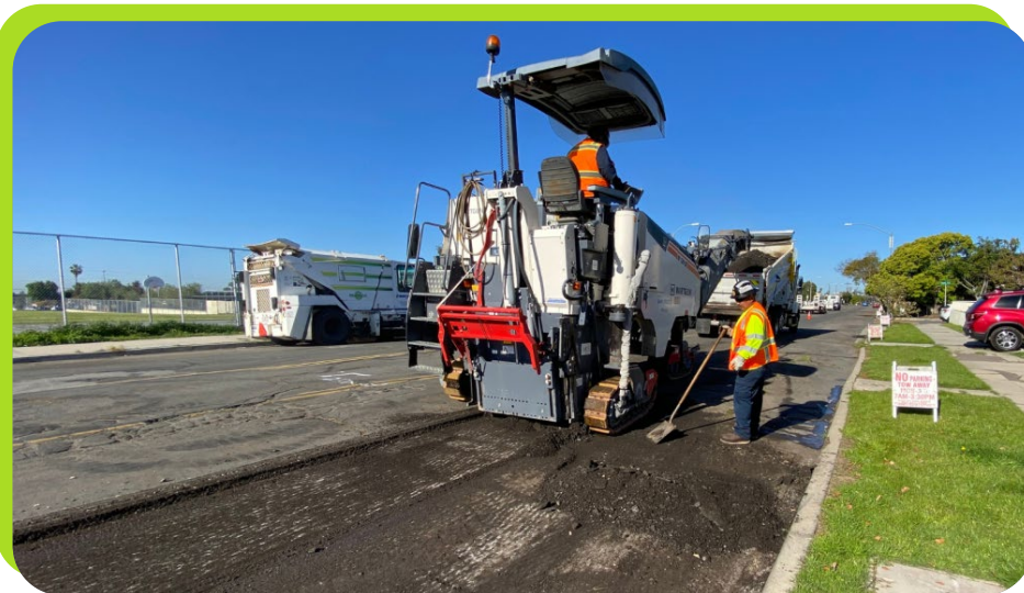
Cold milling operation removing existing pavement surface as part of roadway rehabilitation.
