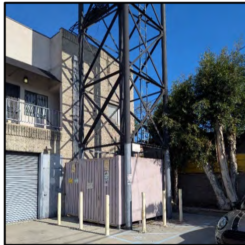
Figure 2 Generator enclosure at the base of the tower
