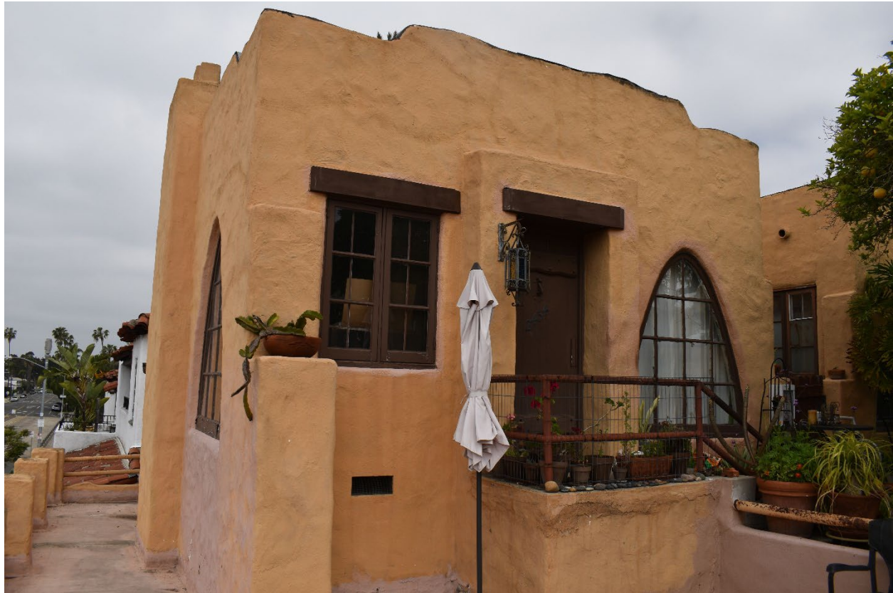
Overview of the east elevation of the westernmost detached bungalow (camera facing northwest)
