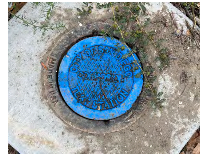
Existing City of San Diego Corrosion test station.
