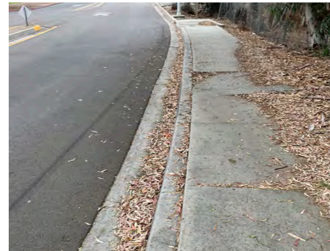
Image shows damage to the existing pedestrian sidewalk running alongside North Mission Bay Road.
