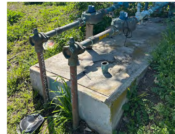
Existing backflow preventer.
