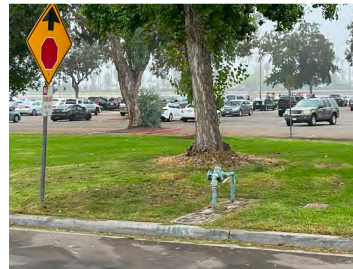
Existing backflow on west side of Mission Bay Drive facing towards the bay.
