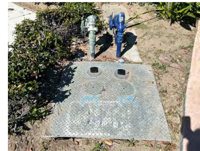
Existing backflow preventer for irrigation system.
