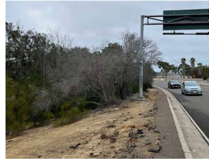
Existing degraded AC pedestrian path.
