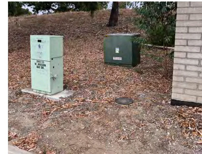
Existing transformer for streetscape irrigation system.
