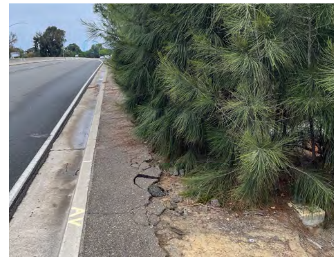
Existing degraded AC paving adjacent to pine grove.
