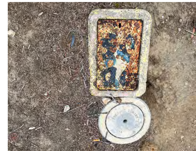
Existing deteriorating irrigation control boxes.
