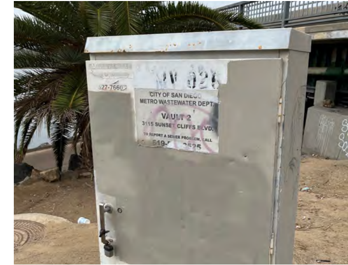
Existing metro wastewater pump station controls.
