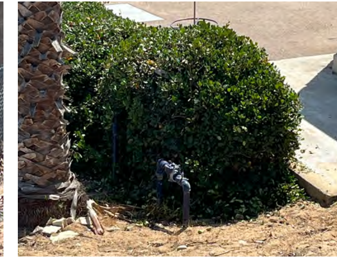
Existing backflow preventer.
