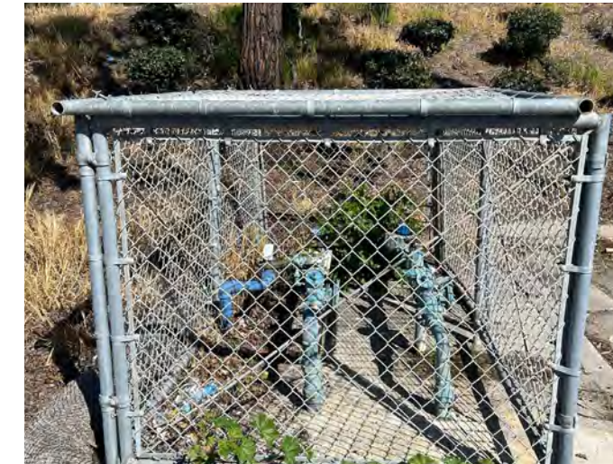
Existing enclosed backflow preventer adjacent to Ingraham Street
