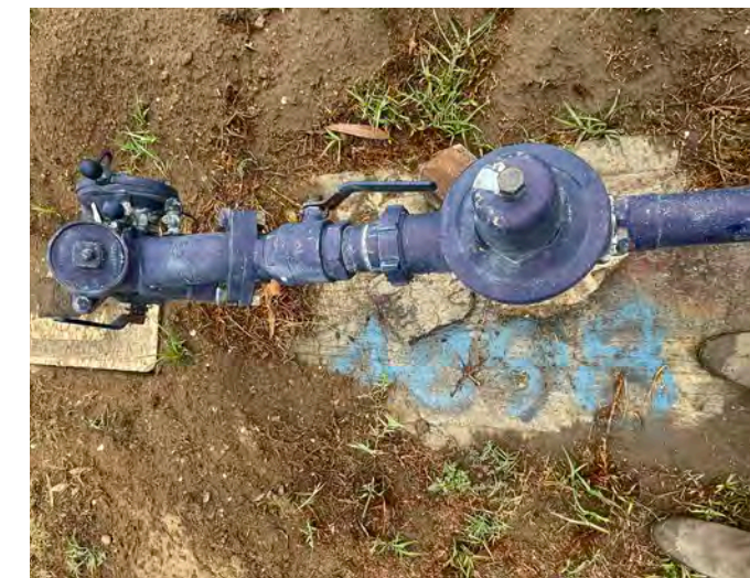
Existing backflow preventer for streetscape irrigation system.
