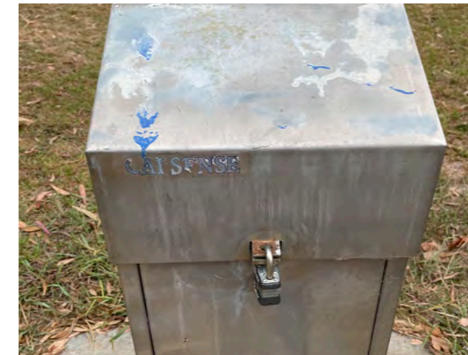
Existing irrigation controller operates open turf area adjacent to golf course.
