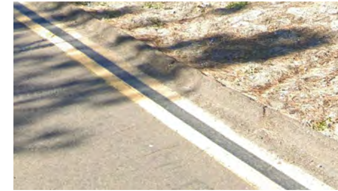
Damaged and undulating curb along the medians on Sea World Drive.
