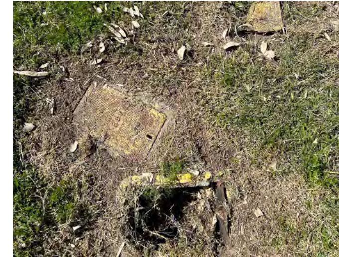
Existing irrigation valve boxes in turf areas.
