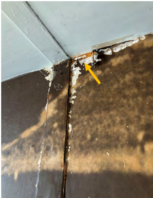
Figure 18: The paper support was severely damaged near the metal joint, as the intrusion of outside air supported pest activity and corrosion (West Wall, before treatment).
