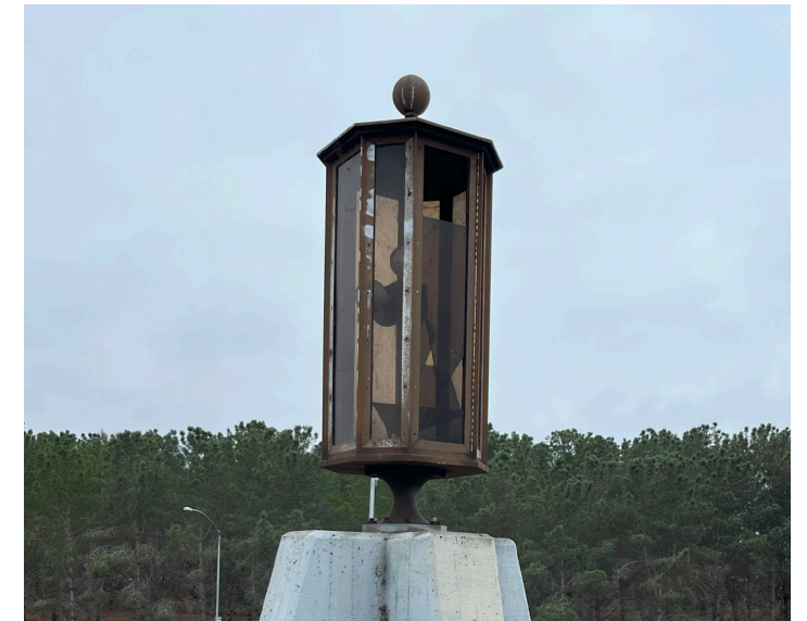
Historical Lantern Repair or Remove with Replicate
