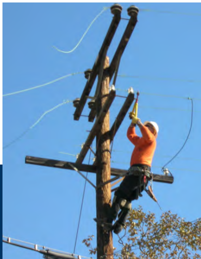
To remove the overhead system, cables are dismantled and removed, and wires are cut.
