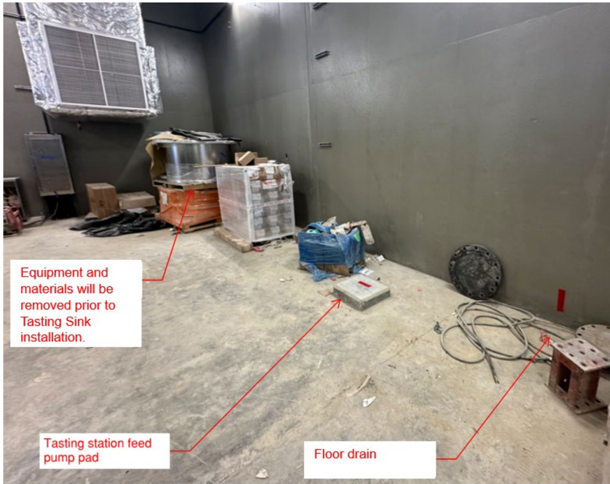
PHOTO #1: TASTING STATION 1 (UV TASTING STATION) SEE ATTACHMENT 4 - TASTING STATION AS-BUILT NOTES.
