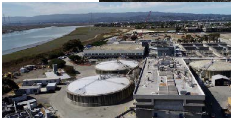
Source Water Facilities at Silicon Valley Clean Water
