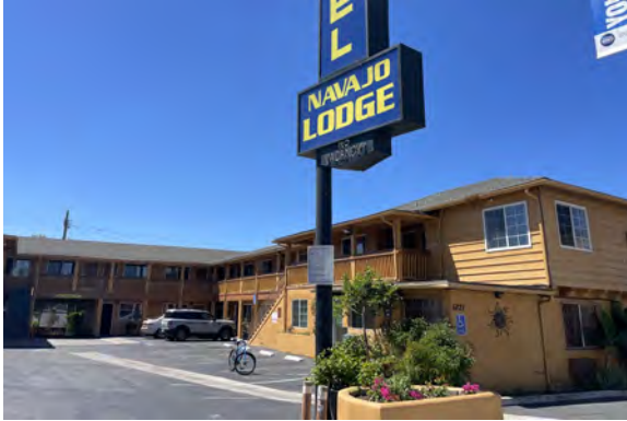
Figure 83: Navajo Lodge (5721 El Cajon Blvd.) motel built c.1950-56 in a Minimal Traditional style. Thematic features such as a teepee and neon signs have been removed, and materials and windows altered.
