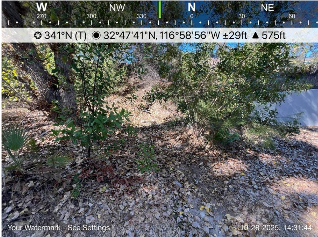
Photo 13. Work Location 439+20, NWW-ALT-05, an ephemeral channel aligned between culvert outfall under West Main Street and flowing toward NWW-ALT-04; facing north. October 28, 2025.
