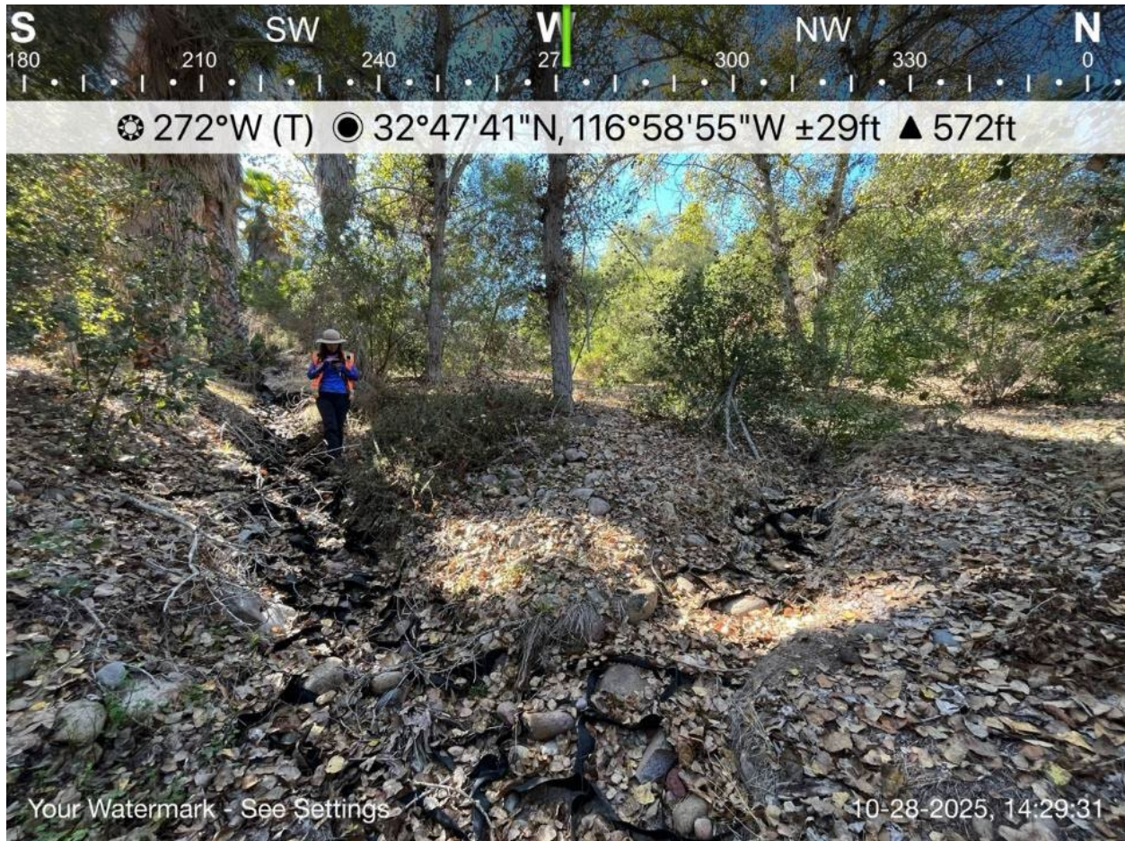
Photo 11. Work Location 439+20. Convergence of ephemeral channel NWW-ALT-04 and intermittent channel NWW-ALT-05; both provide surface flow connections to stormwater culverts. Note existing geogrid and rock installed to reduce erosion. View facing west. October 28, 2025.
