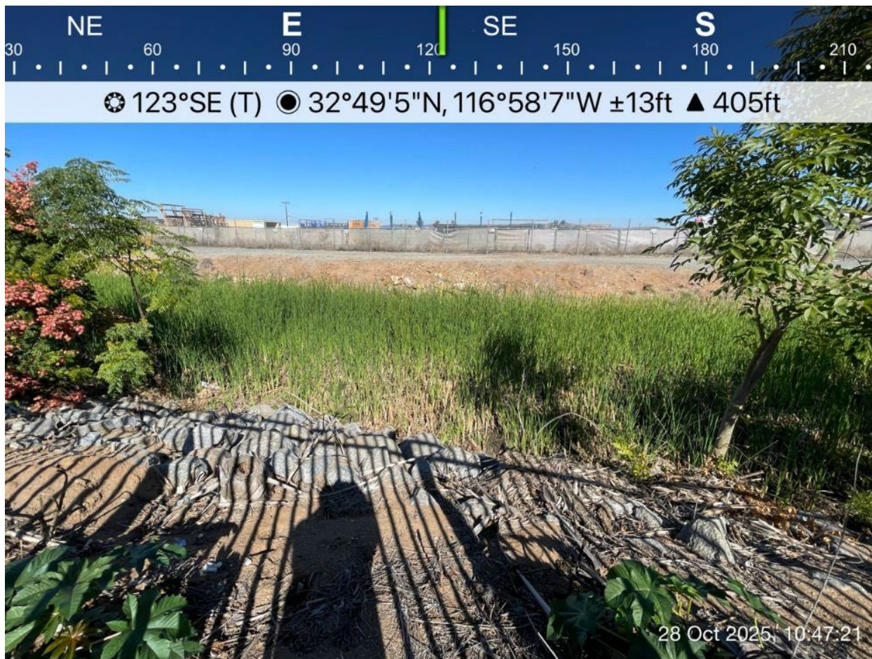
Photo 3. Work Location 345+20 and a view of NWW-ALT-01, a canal constructed between W Bradley Avenue and Floyd Smith Drive; facing southeast. October 28, 2025.
