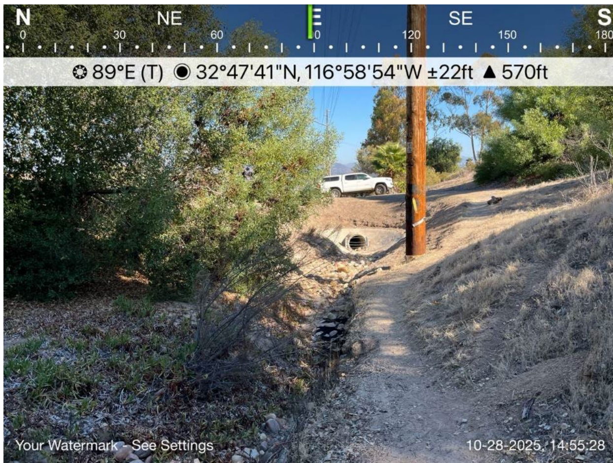
Photo 10. Work Location 439+20, NWW-ALT-04; view of culvert inlet that directs water from both NWW-ALT-04 and -05 into an underground stormwater system of pipes that are assumed to flow 0.75-miles to a channelized reach of Forester Creek; View facing east. October 28, 2025.
