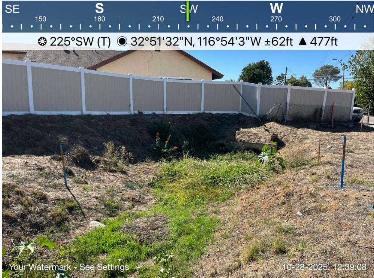
Photo 8. Adjacent to work location at 40+29, NWW-ALT-03 is a drainage feature with soil substrate. View facing southwest. October 28, 2025
