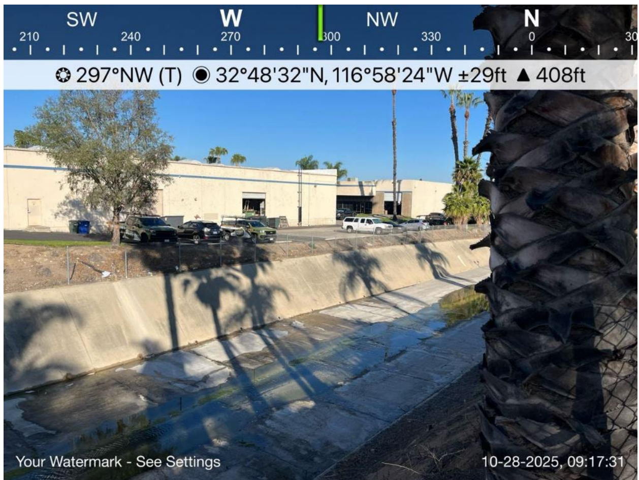
Photo 4. Work Location 380+15 and a view of NWW-ALT-02, a channelized waterway; facing west. October 28, 2025.
