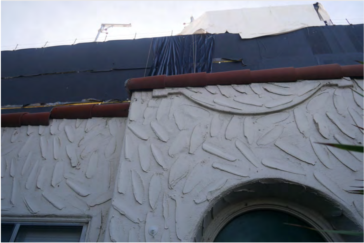
Photograph #24: Non-original heavy textured stucco
