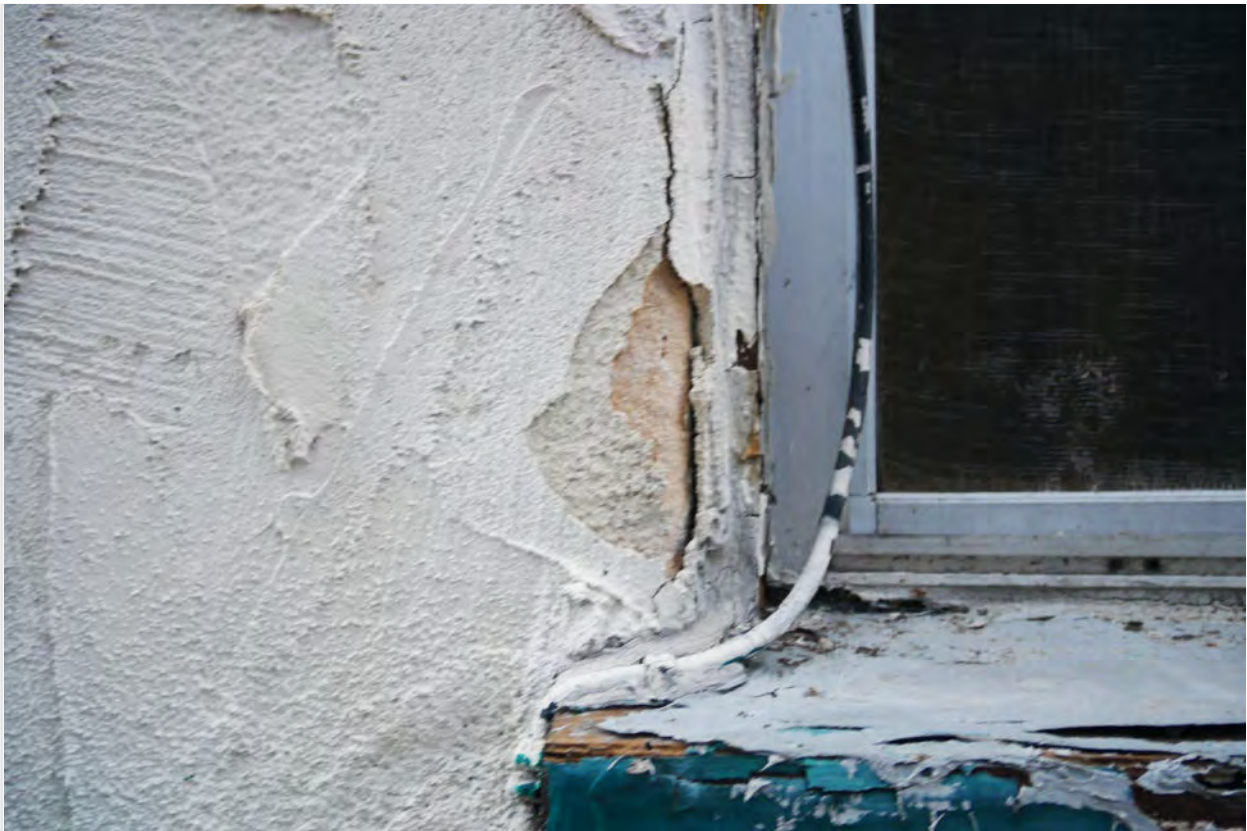
Photograph #71: Non-original heavy textured stucco failing and exposed original stucco texture visible
