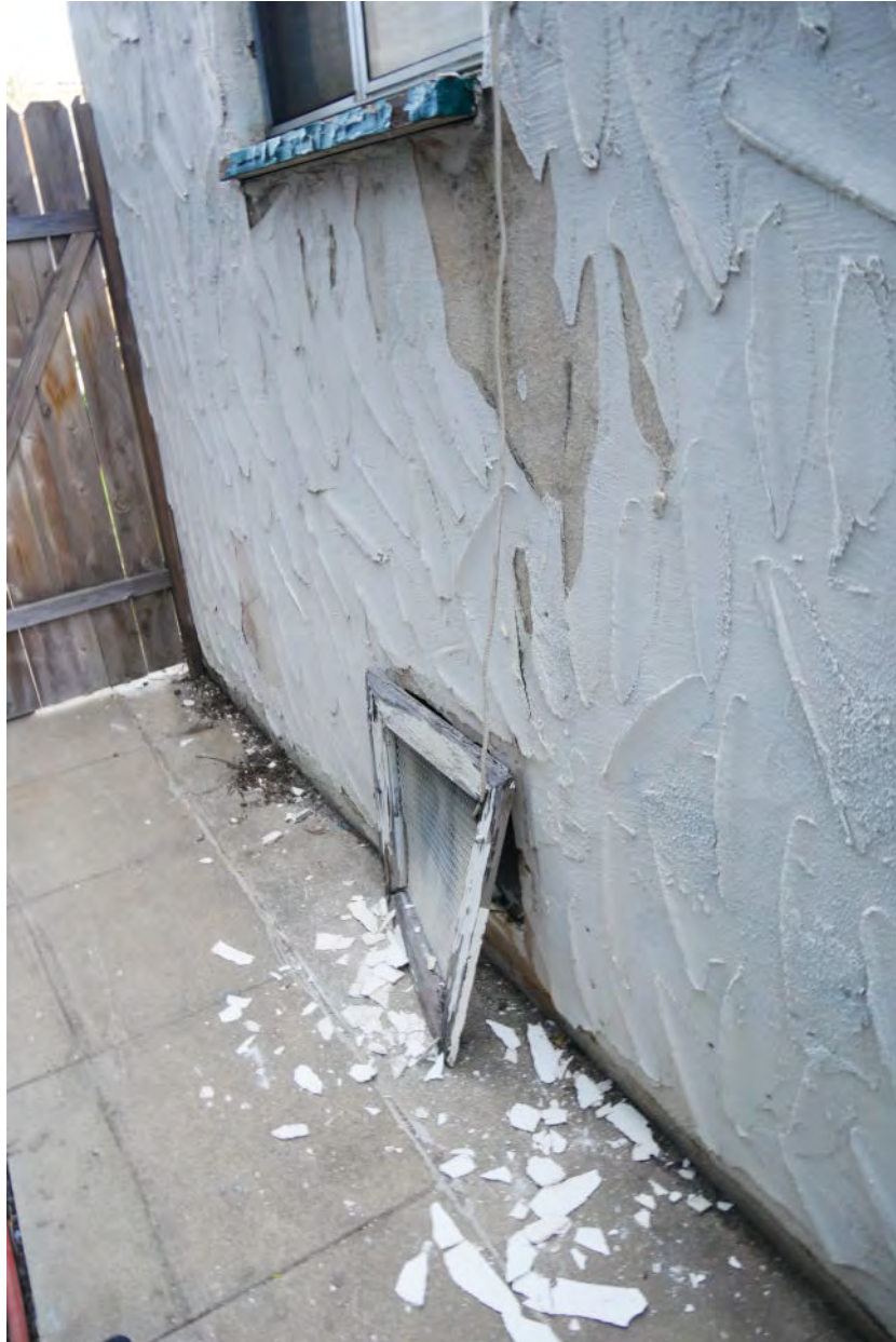
Photograph #60: Non-original heavy textured stucco failing and exposed original stucco texture visible
