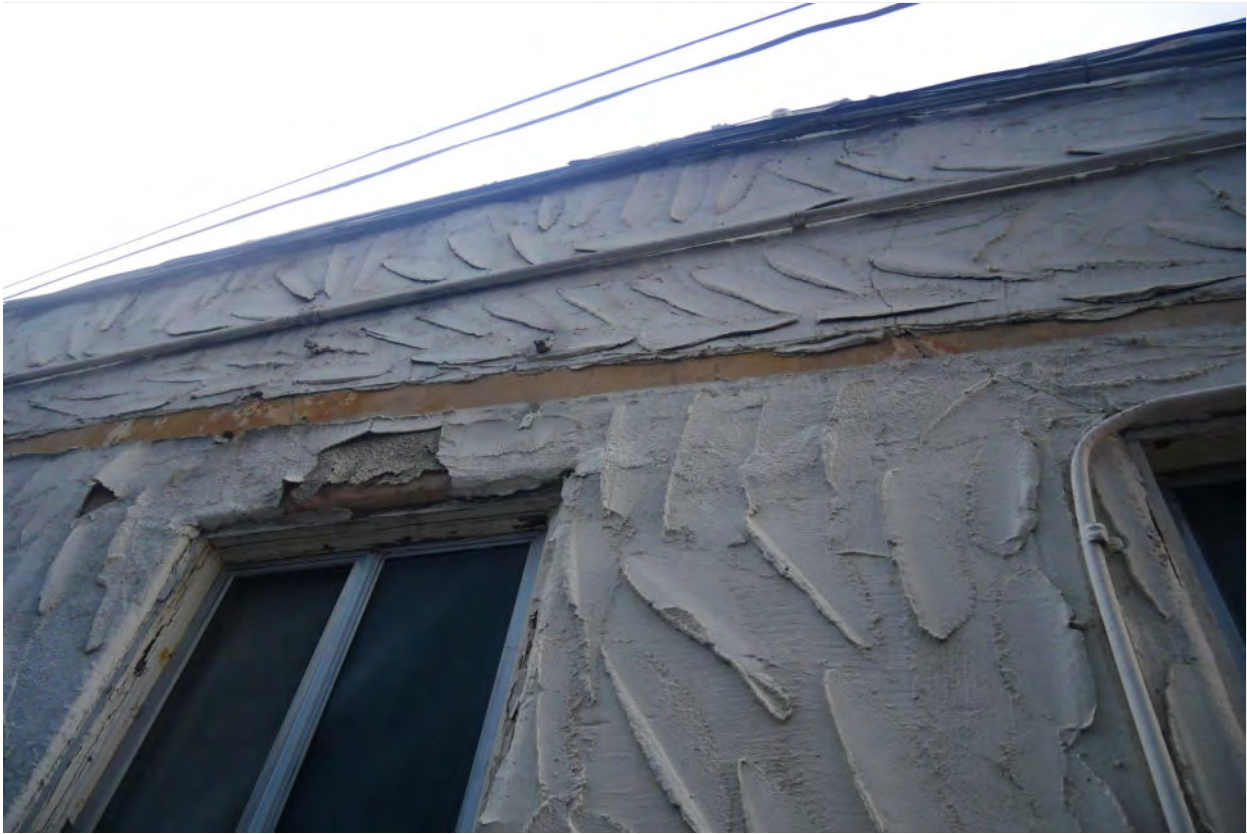
Photograph #26: Non-original heavy textured stucco
