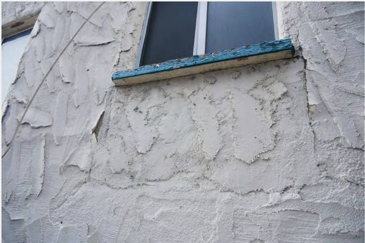
Photograph #50: Non-original heavy textured stucco failing with patched area
