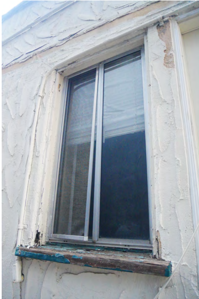
Photograph #28: Typical metal slider window and non-original heavy textured stucco
