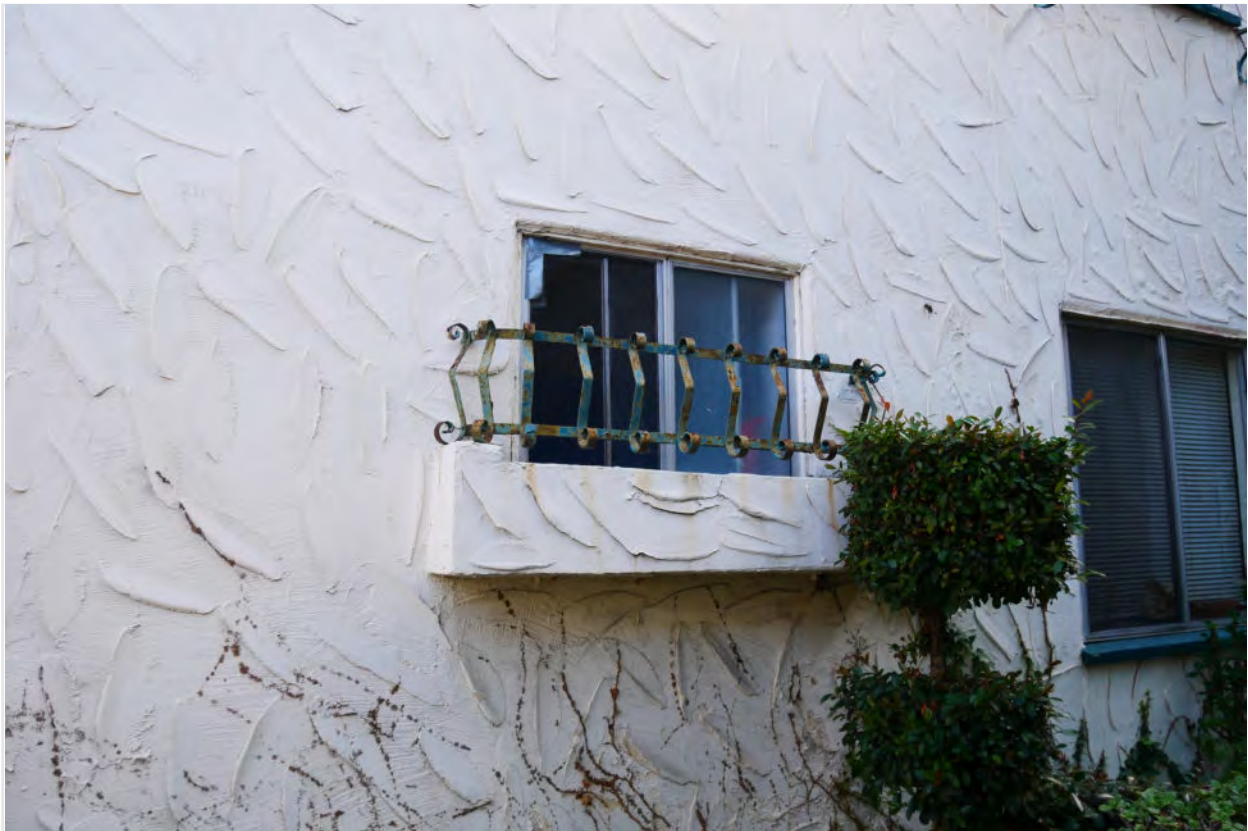
Photograph #38: Heavy textured non-original stucco and metal slider windows, typical all window openings.
