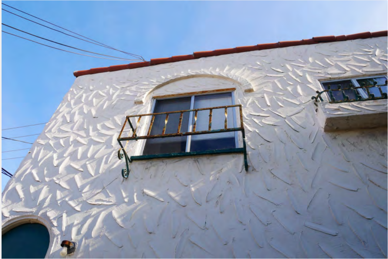
Photograph #37: South elevation two story duplex with rusted wrought iron
