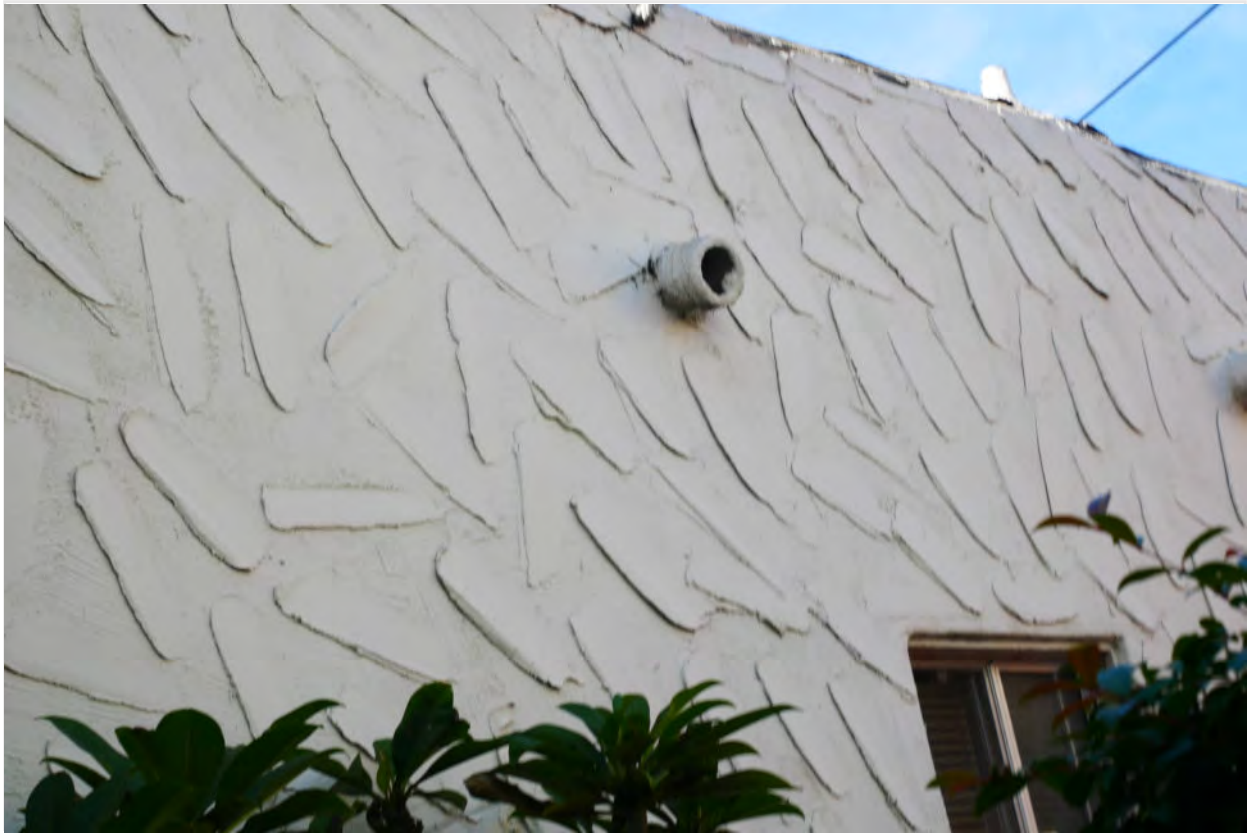
Photograph #81: Non-original heavy textured stucco
