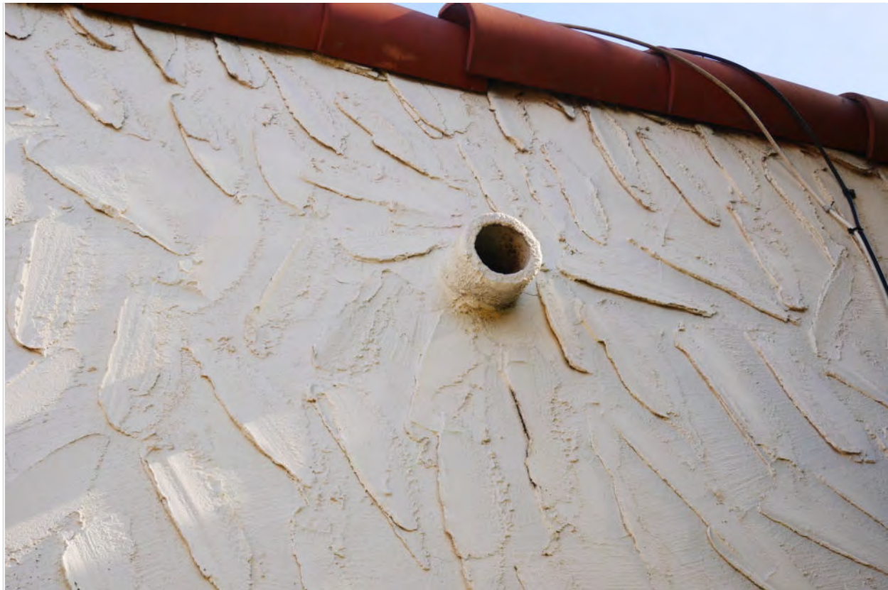
Photograph #82: Non-original heavy textured stucco
