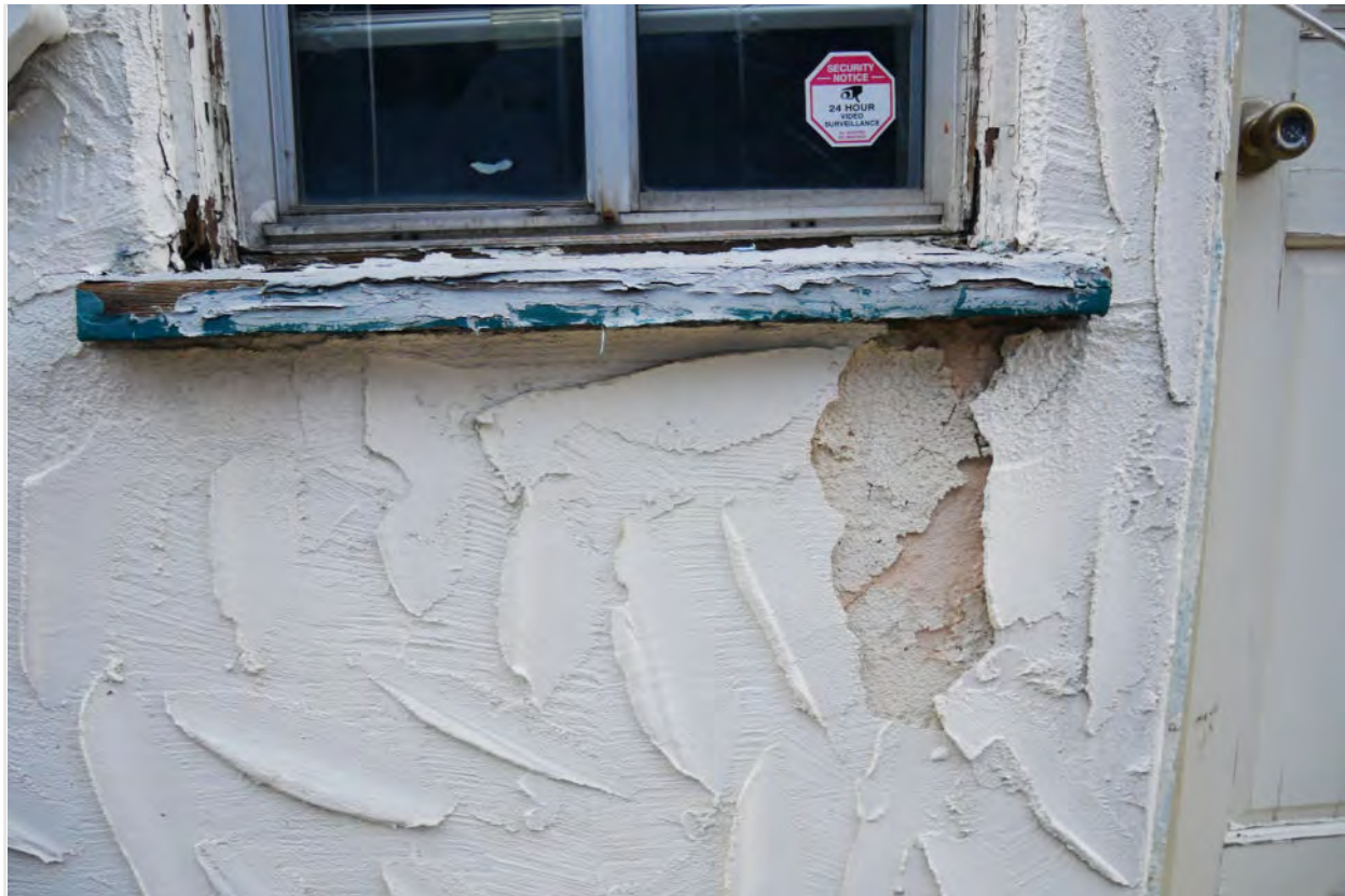
Photograph #27: Non-original heavy textured stucco
