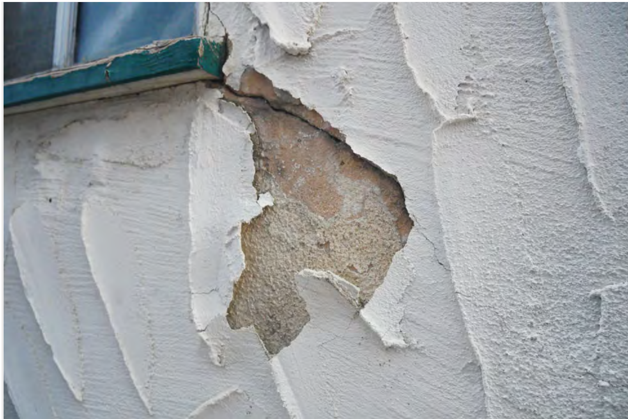
Photograph #25: Non-original heavy textured stucco
