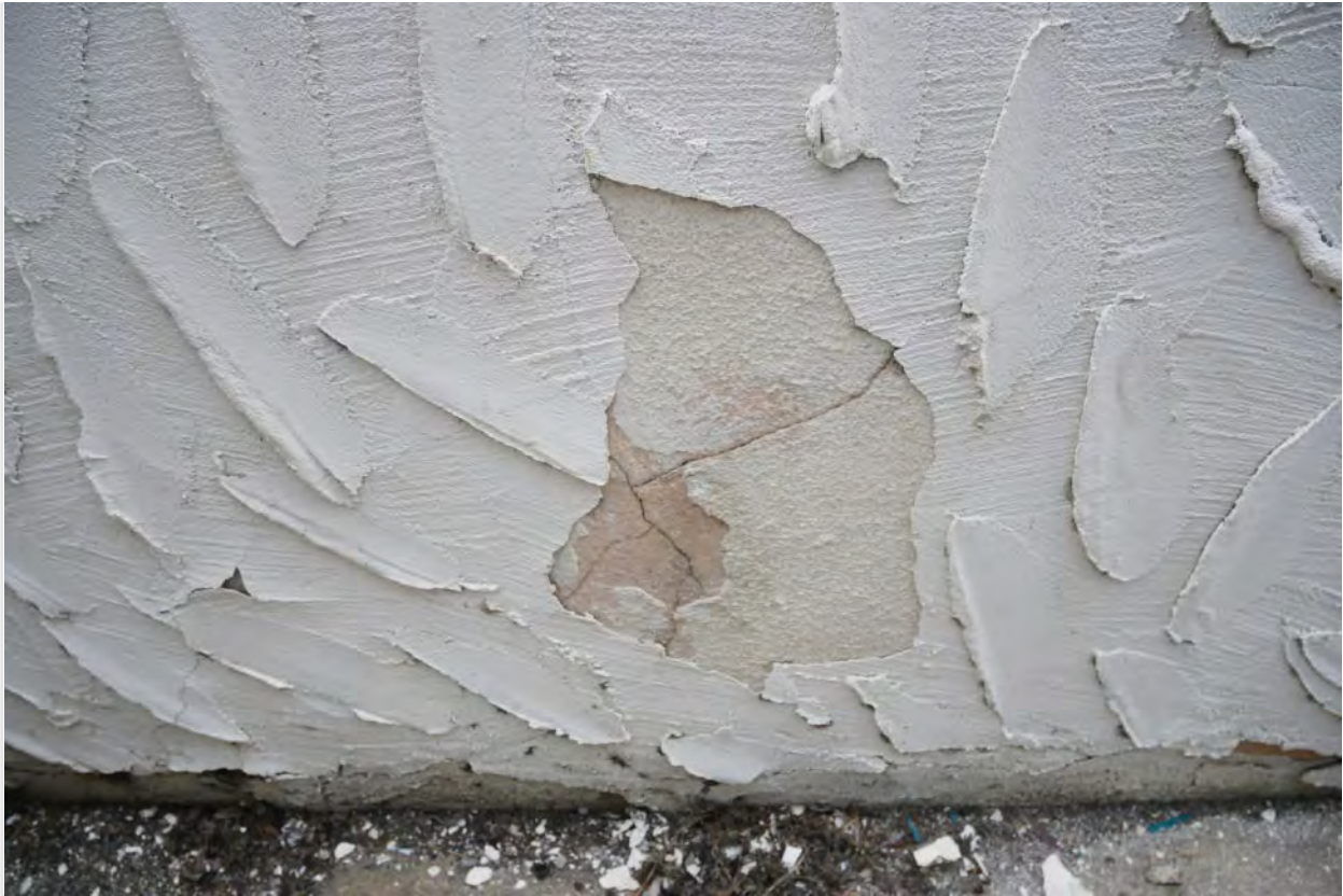
Photograph #70: Non-original heavy textured stucco failing and exposed original stucco texture visible
