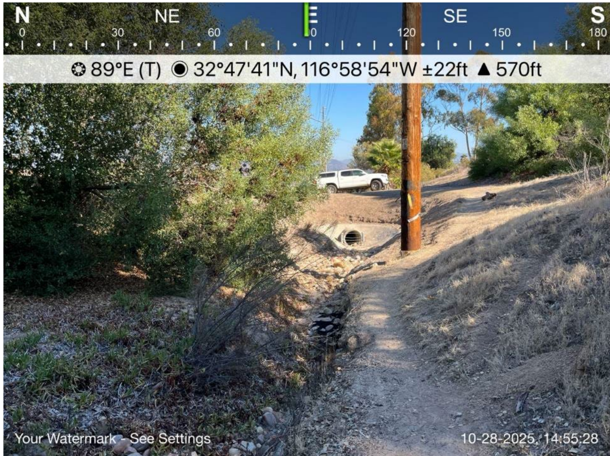
Photo 8. Work Location 439+20, NWW-ALT-04; view of culvert inlet that directs water from both NWW-ALT-04 and -05 into an underground stormwater system of pipes that are assumed to flow 0.75-miles to a channelized reach of Forester Creek; View facing east. October 28, 2025.
