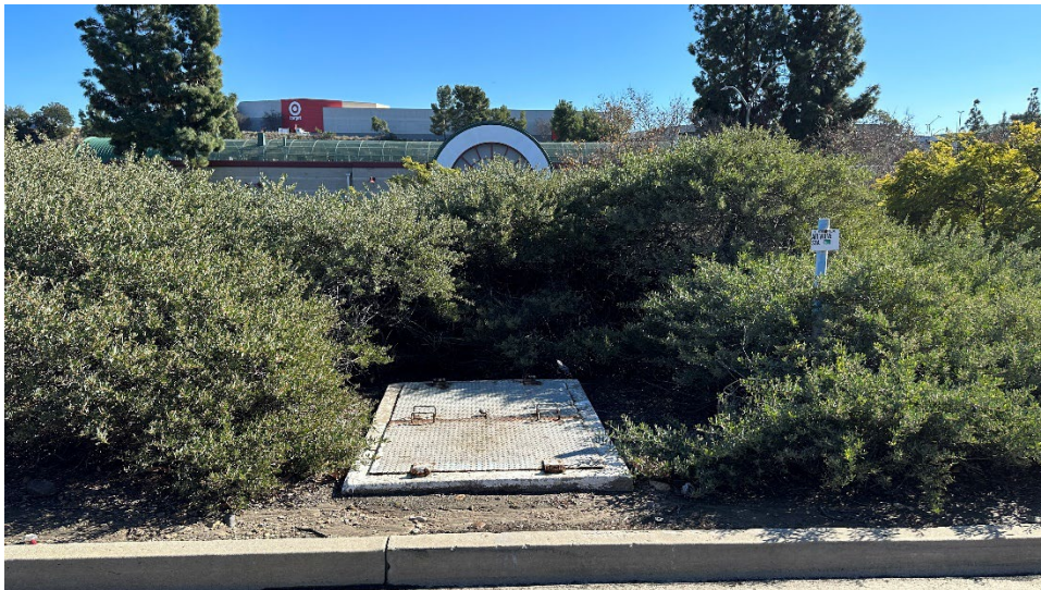
Figure 14. 561+33, Overview of ISO Valve, facing southeast.
