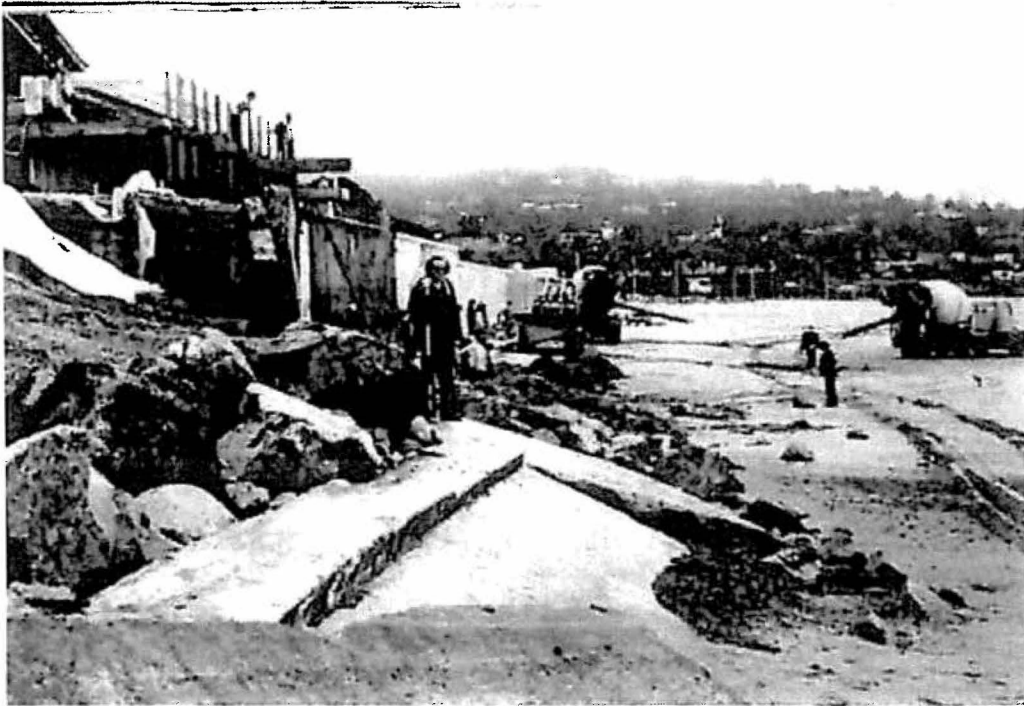
Photo #5: Same location as Photo #2-#5, showing partial collapse of seawall in 1978 (Kuhn, 1984)
