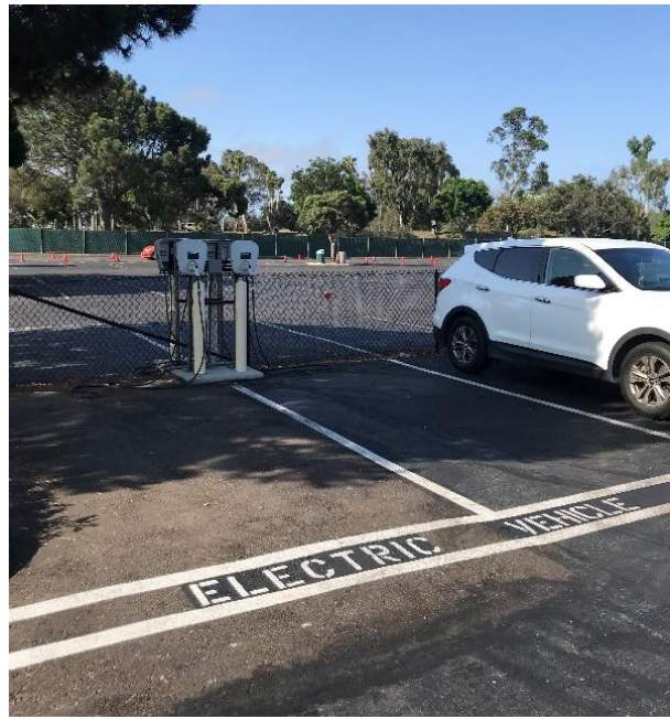
Electric vehicles charging stations
