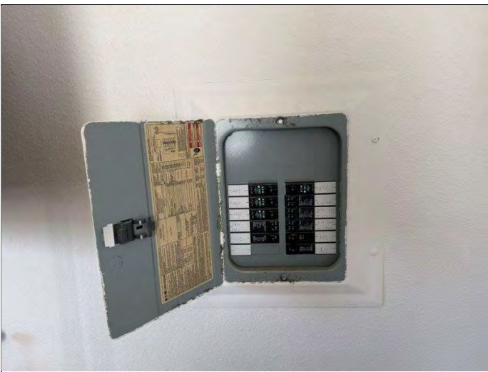
29. Typical unit breaker panel.
