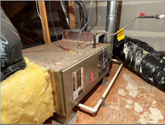
25. Forced heat furnace at attic of unit 1556.
