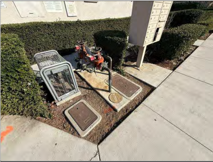
19. Domestic water meter and backflow cage and fire water backflow.
