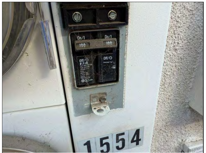
30. Typical unit main breaker service rating of 100 amps.
