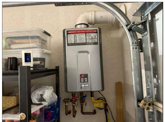
24. Unit tankless water heater in garage of 1556 residence.
