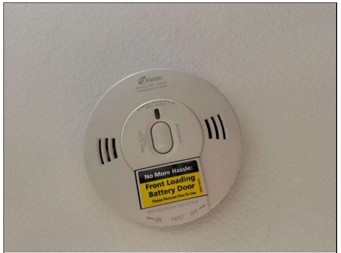
28. Typical unit smoke and carbon monoxide detector.
