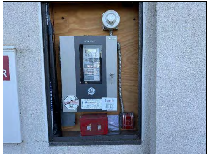
22. Fire alarm panel at 1556-1558 Building.
