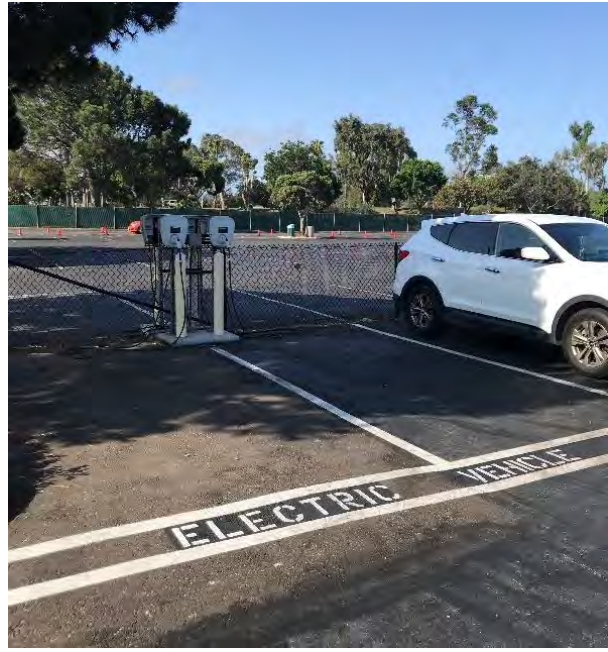
Electric vehicles charging stations
