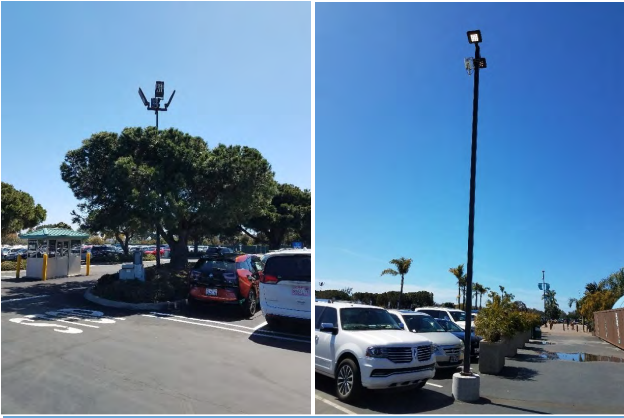
Typical parking lot lighting
