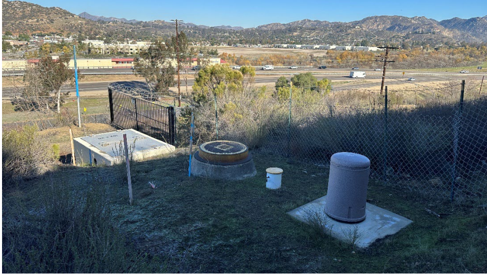
Figure 3. 187+35, Overview of ISO Valve within APE, facing north northwest.
