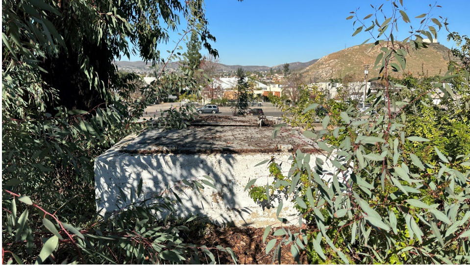
Figure 5. 226+29, Overview of ISO Valve, facing northwest.
