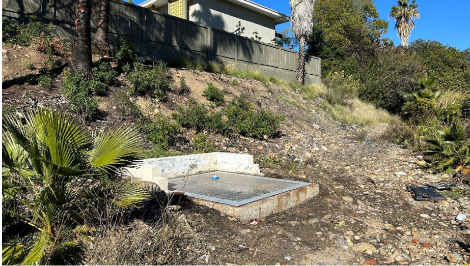
Figure 13. 555+79, Overview of ISO Valve, facing north.
