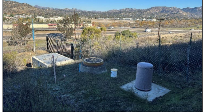
Photo 2. Overview of "ISO valve." View facing north-northwest.
