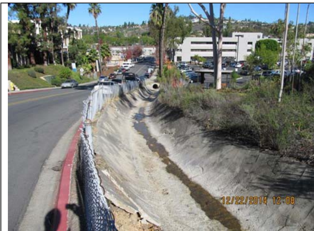
Photo 7: Downstream (facing north) looking toward inlet pipe, approximate location of Photo 3, December 22, 2014.
