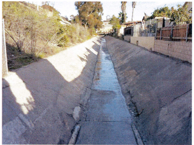
Photograph 10: Upstream view from 3094 Via de la Bandola of channel after emergency maintenance.
