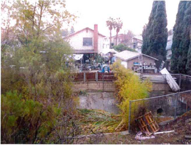
Photograph 5: On the north side of the channel looking south to 3094 Via de la Bandola – This photo was taken on 12.3.14. The leaning tree has been observed by the crews to have worsened over time.
