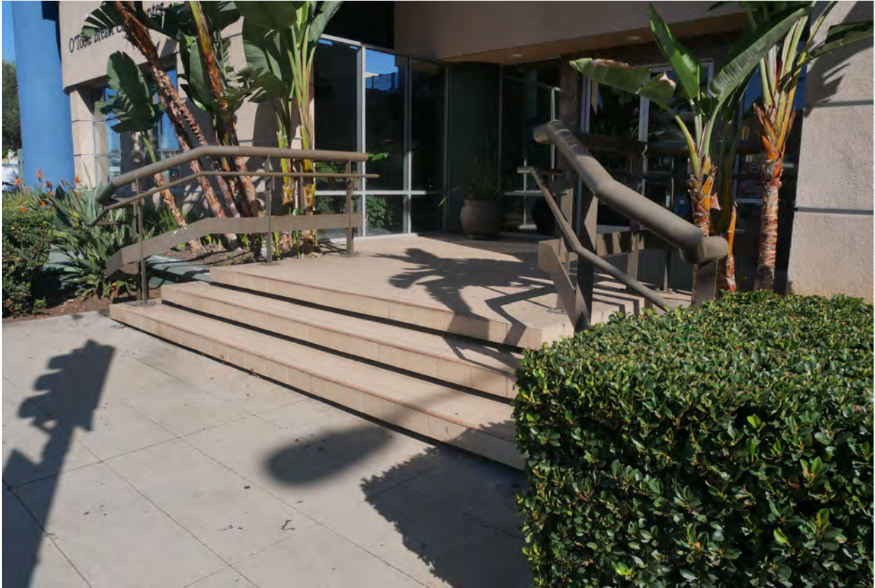
Photograph #15: Front entry. Original bridge removed and new entry with stairs and guardrails added 2003.
