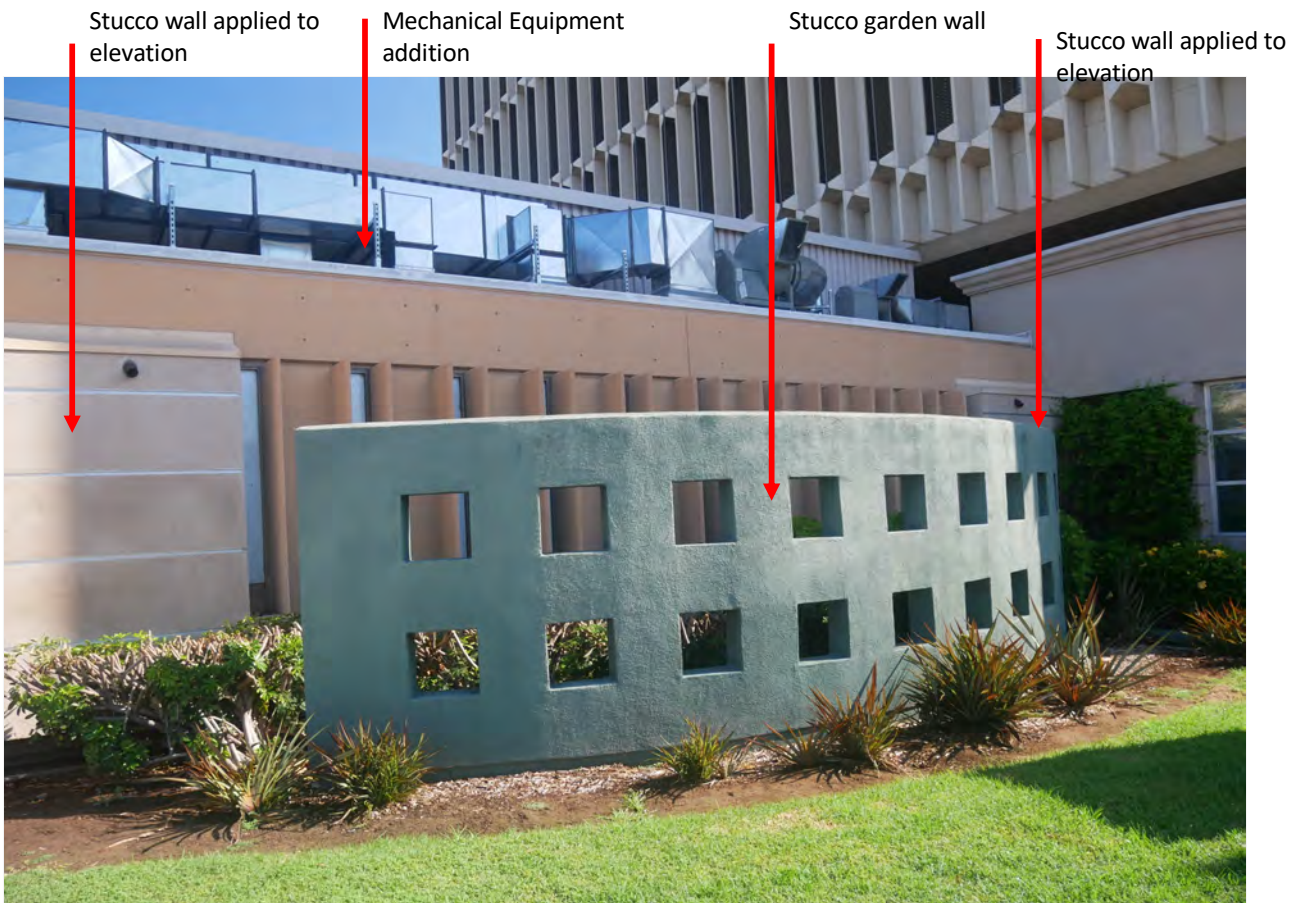
Photograph #20: Front, Garden wing walls and stucco walls added to one story wings and mechanical units on roof.
