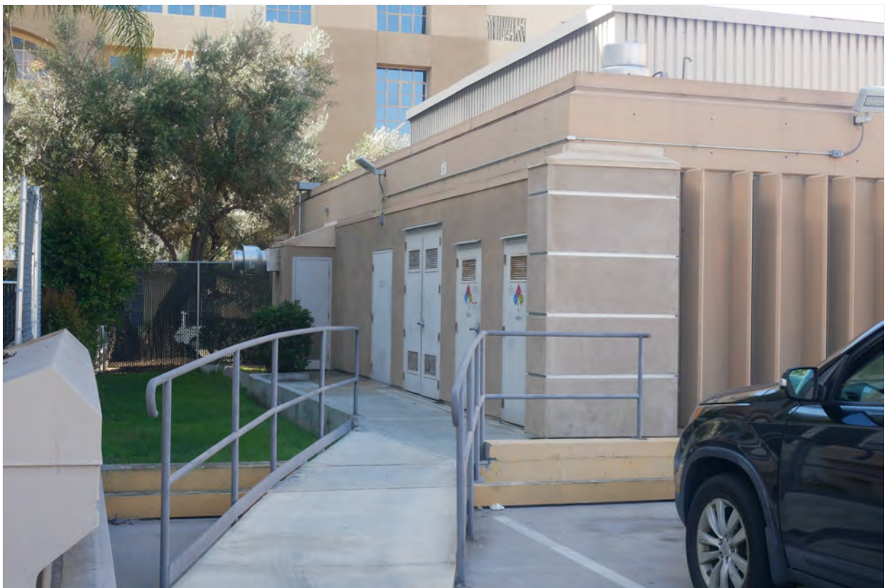
Photograph #30: East elevation with stucco infill and mechanical addition on roof.
