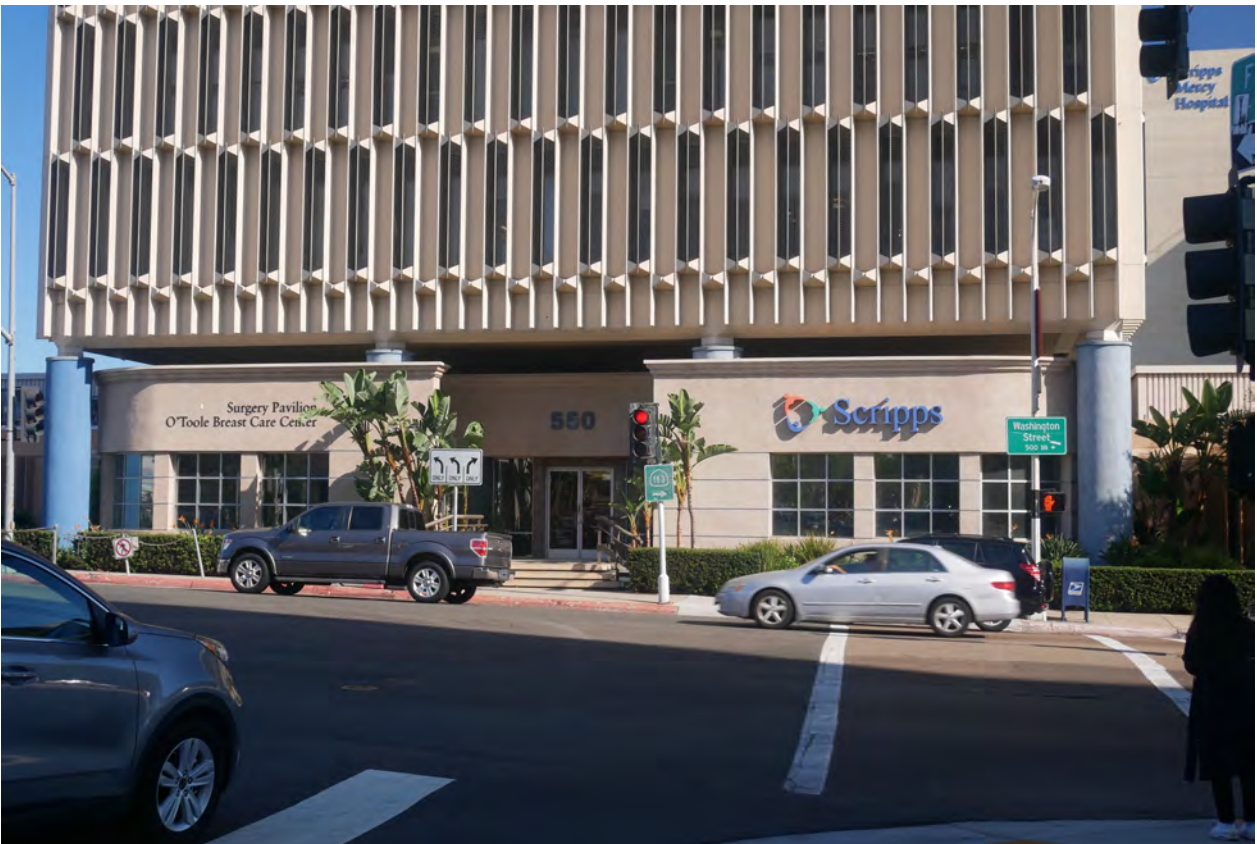
Photograph #14: Front, South elevation. Changes: Lobby is completely enclosed with stucco walls, aluminum storefront system and round column enclosures. Stucco garden walls block one-story wings. Mechanical additions on top of wings and bridge entry into lobby is gone.
