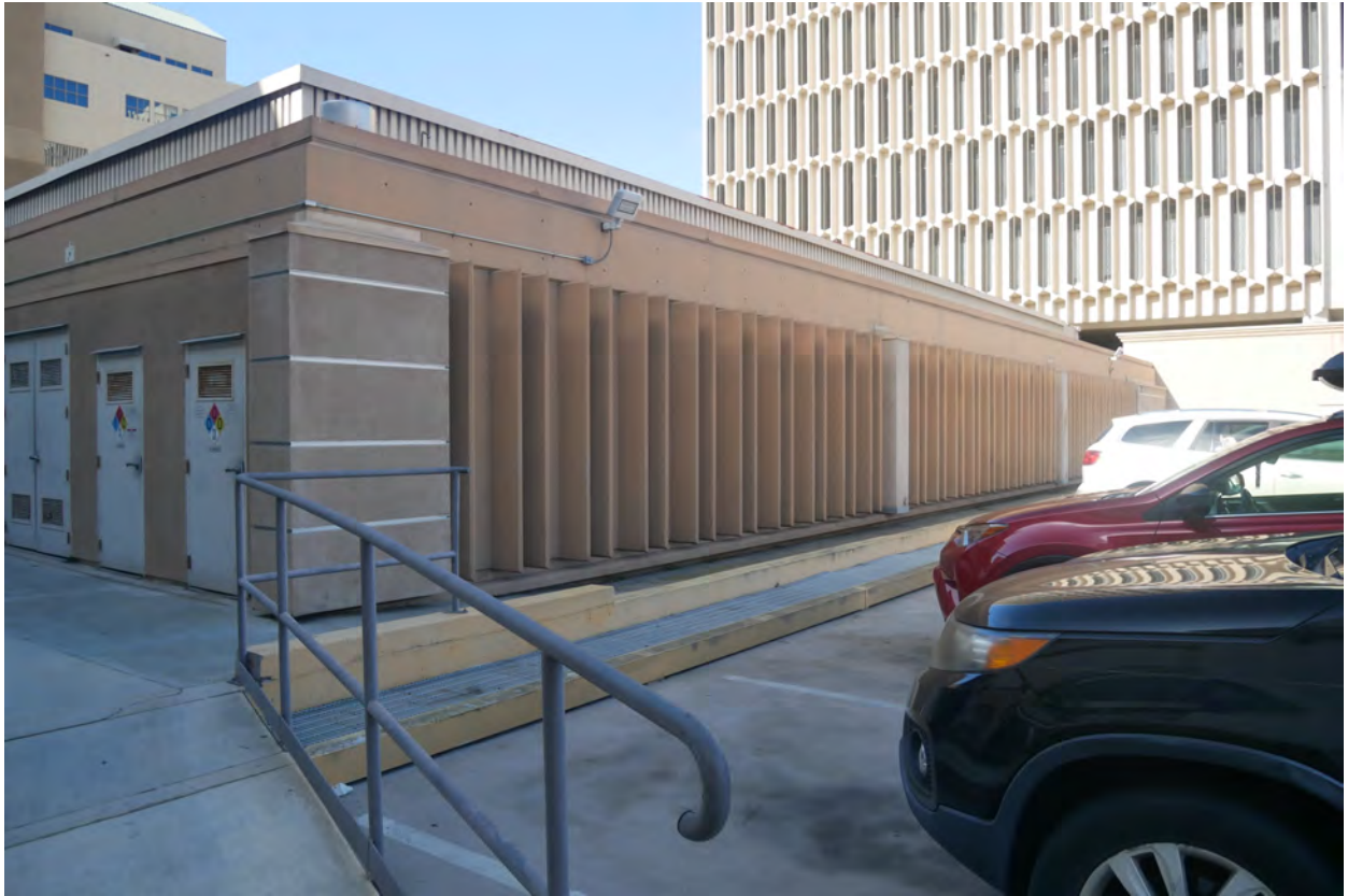
Photograph #29: Northeast elevation. One-story east wing, with stucco infill at east end and mechanical addition on roof.
