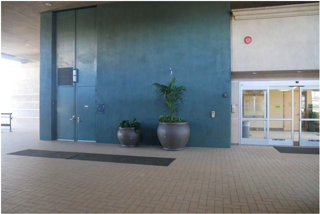
Photograph #34: Lobby interior. All original materials – paving and marble (specially ordered charcoal brown marble sourced from Italy) are no longer extant.
