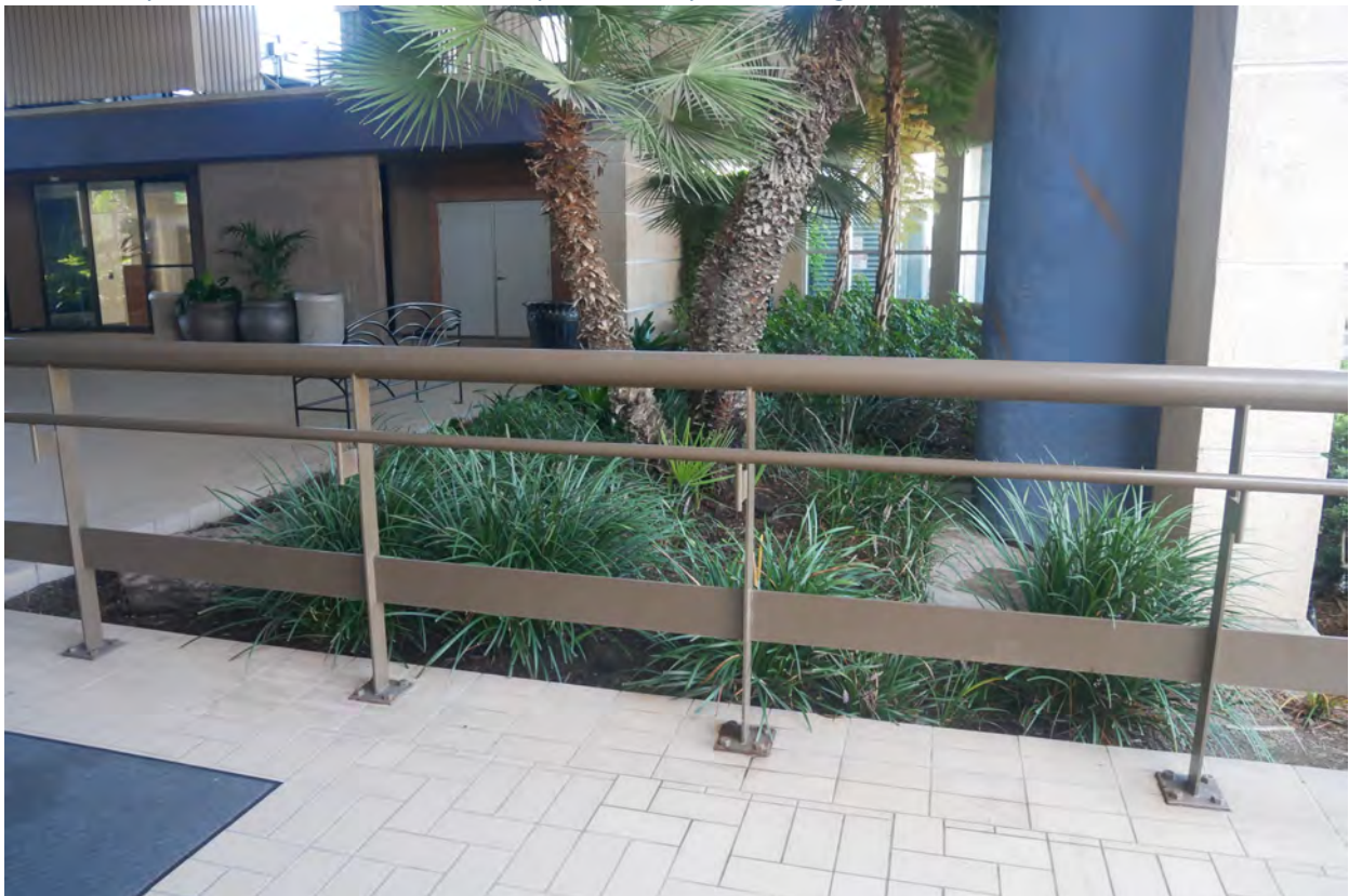
Photograph #33: Former open-air lobby and reflecting pool. New walkway and landscaping removed original bridge and (4) pools. Columns were enclosed with round stucco enclosures. Stucco infill can be seen on one-story wing with mechanical addition on roof.
