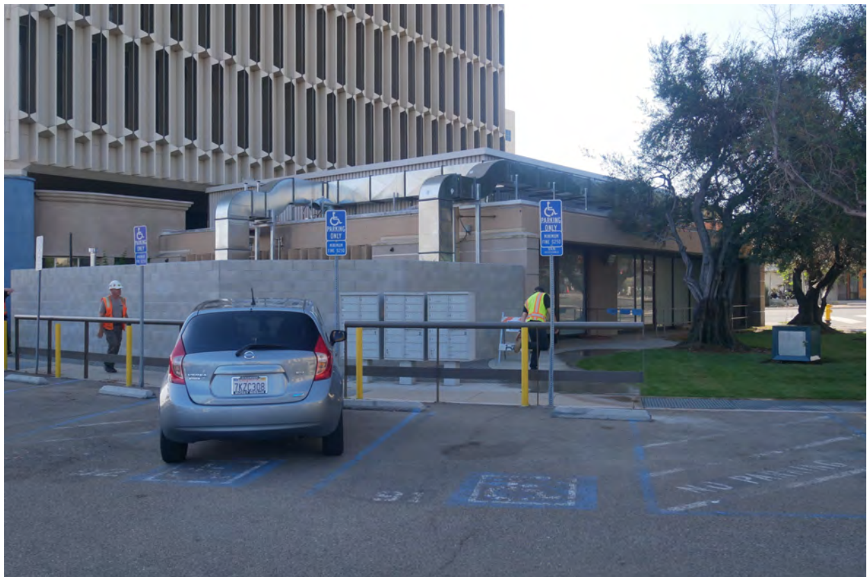
Photograph #22: Rear, north elevation. One-story wing with mechanical units and block wall enclosure for generator, 2003.
