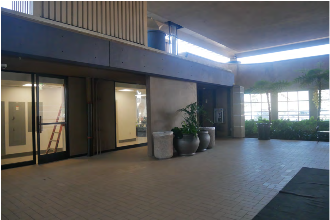
Photograph #35: Former open-air lobby. East elevation of one-story wing with visible mechanical units and stucco infill. Stucco garden wall and aluminum dual glazed windows enclose lobby along north side of lobby.
