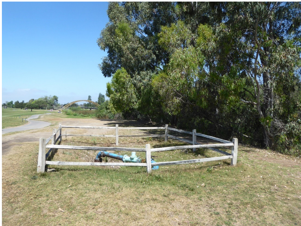
Figure 69. A pump/lift station near the first hole of the Mission course. Photograph taken facing west.
