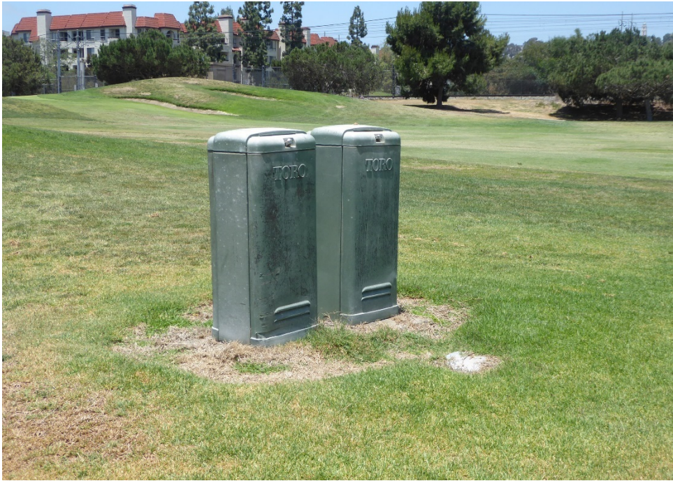
Figure 70. Example of TORO irrigation boxes on the fourth hole of the Presidio course. Photograph taken facing west.
