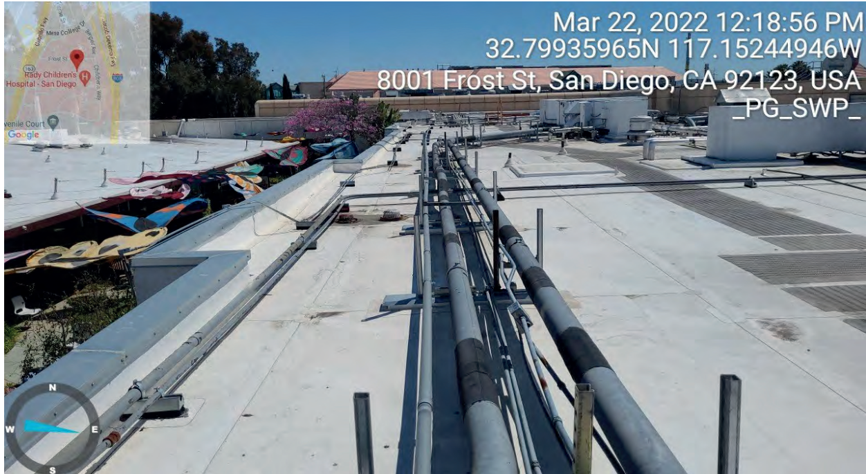
View east of piping towards the Medical Office Building on the roof of the Hanh Pavilion located on the northeast portion of the Project boundary.
