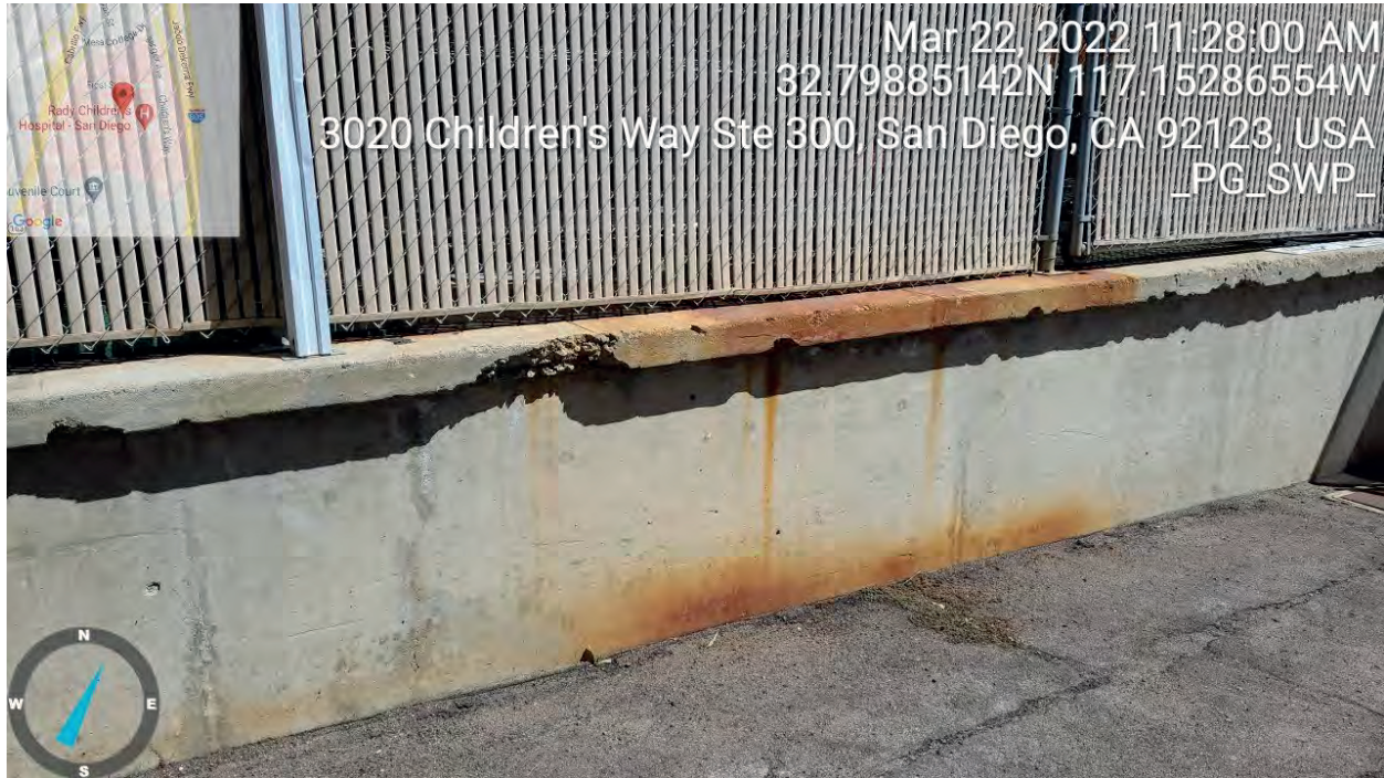
View northeast outside Building 12 located on the west portion of the Project boundary. Area contains rust stains on the concrete.
