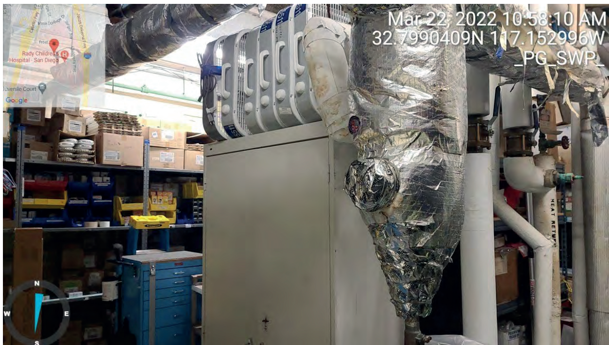
View southwest inside a carpenter room on the second floor of Building 12 located on the west portion of the Project boundary. Area contains asbestos per sign posted on door.
