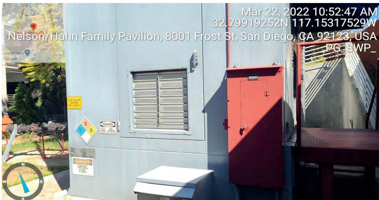
View northwest toward a generator located on the west portion of the Project boundary.
