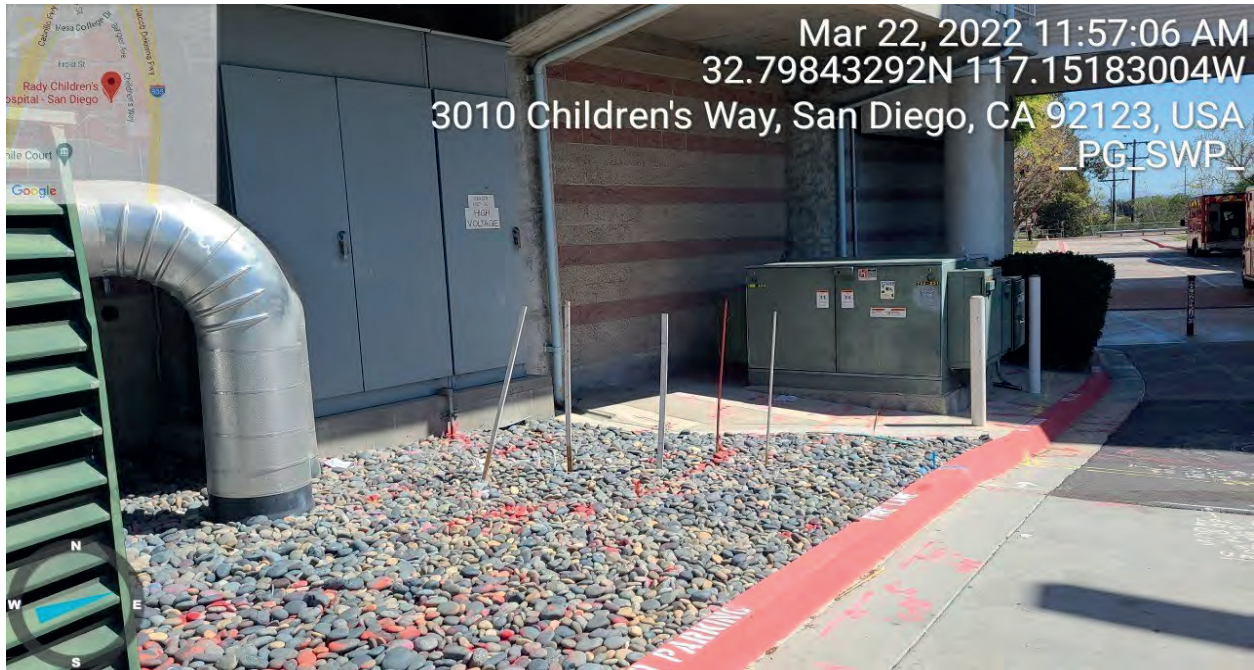
View northeast toward electrical transformers outside the Hanh Pavilion located on the central portion of the Project boundary.
