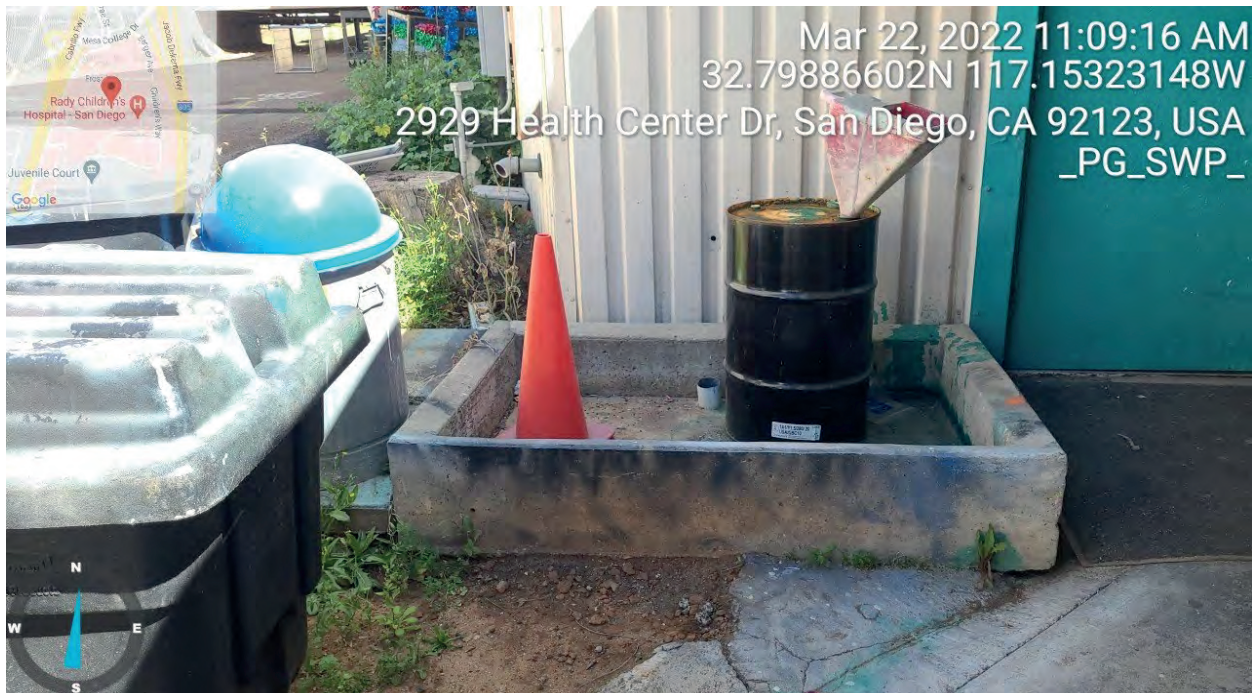
View north outside a paint room on the first floor of Building 12 located on the west portion of the Project boundary. The 55-gal. drum likely contains leftover paint stored outside in cement drainage basin; the basin was observed to have residual paint spills and markings.
