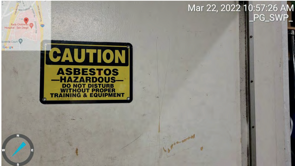
View southwest inside a carpenter room on the second floor of Building 12 located on the west portion of the Project boundary. Area contains asbestos per sign posted on door.
