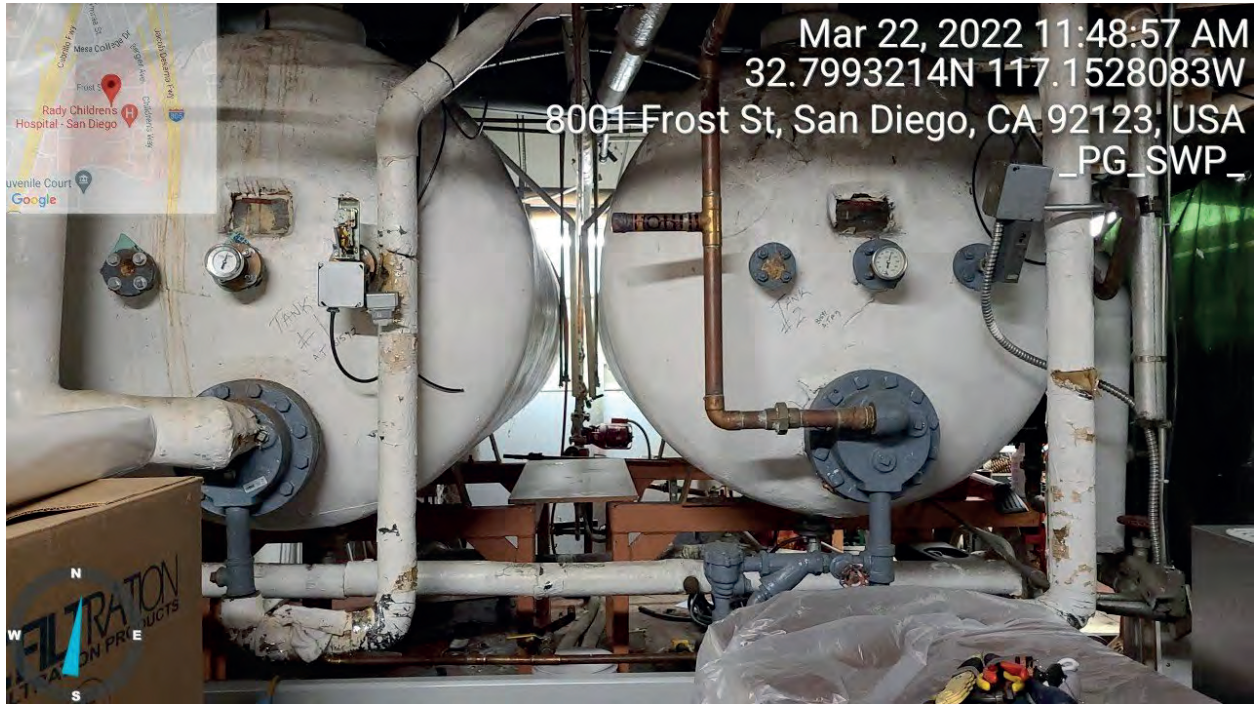
View north in a room located on the second floor of Building 12 located on the west portion of the Project boundary. Area contains two water tanks connected to a piping system; area also stores chemicals and gas tanks.
