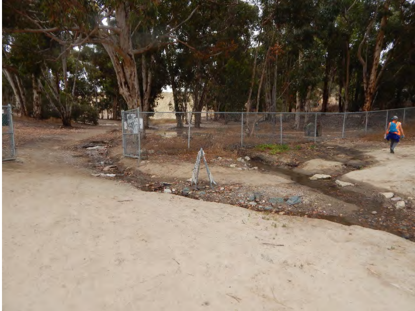
Photo 14. Overview of directed waterflow at Dam gate, The Weir is located in the background at base of slope. View to the southeast.
