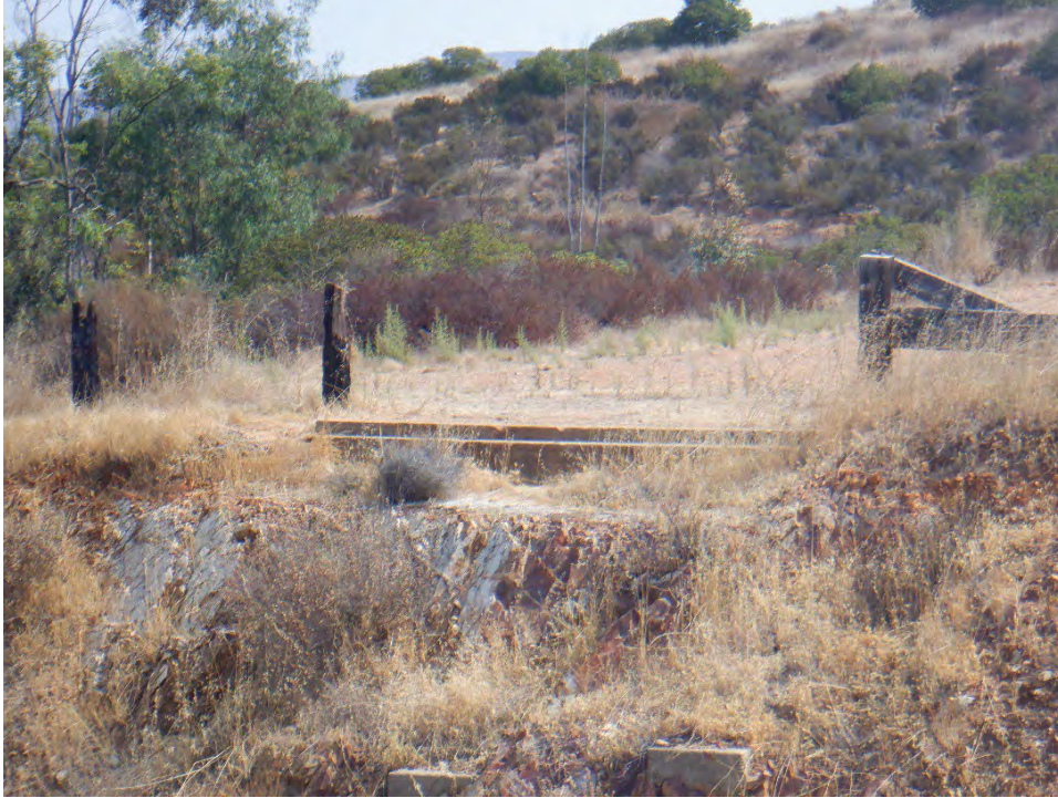
Plate 31. Concrete approach slab and wooden posts and fence remnants on the east side of the spillway, looking northeast.
