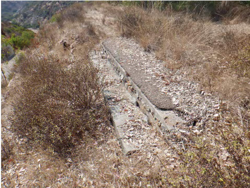
Plate 30. Close up of concrete approach slab with layer of rocks and a top layer of asphalt, looking southeast.
