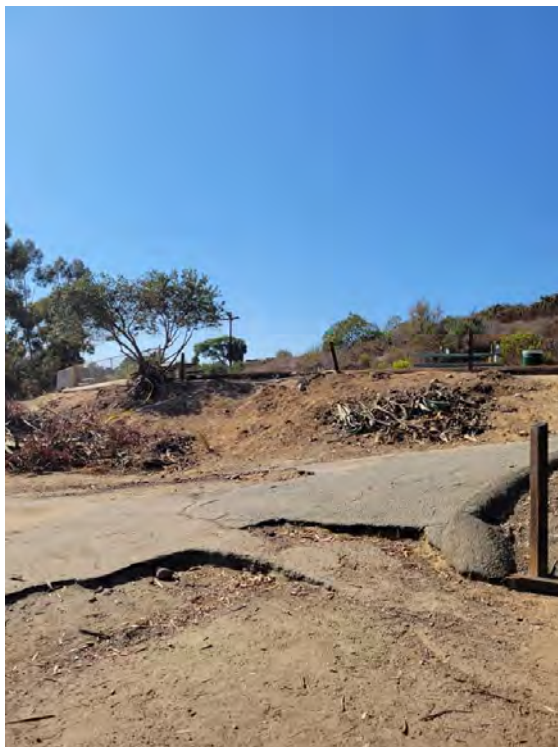
Photo 8. Remnants of concrete along earthen embankment. Looking west towards parking lot.
