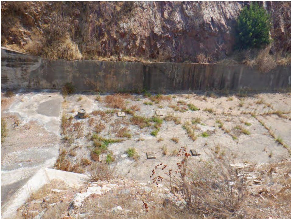
Plate 32. Concrete bridge pier remnants extant on the concrete floor of the spillway, looking east.
