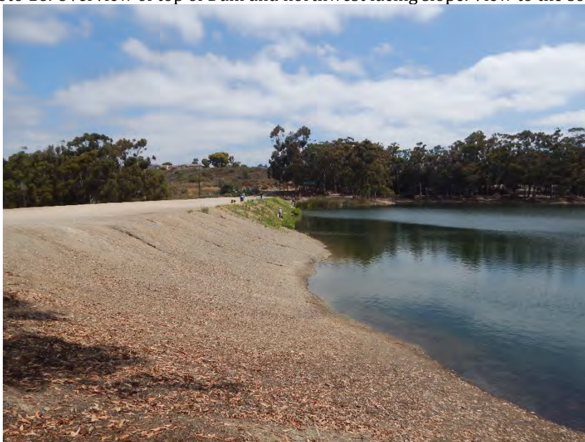
Photo 17. Overview of top of Dam and southeast slope to lake. View to the northeast.
