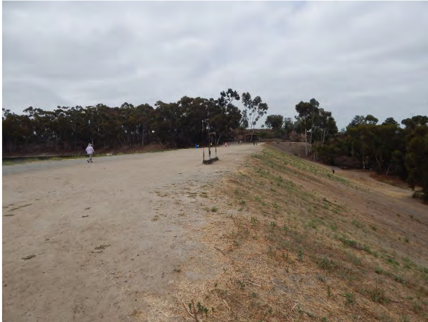
Photo 16. Overview of top of Dam and northwest facing slope. View to the south.
