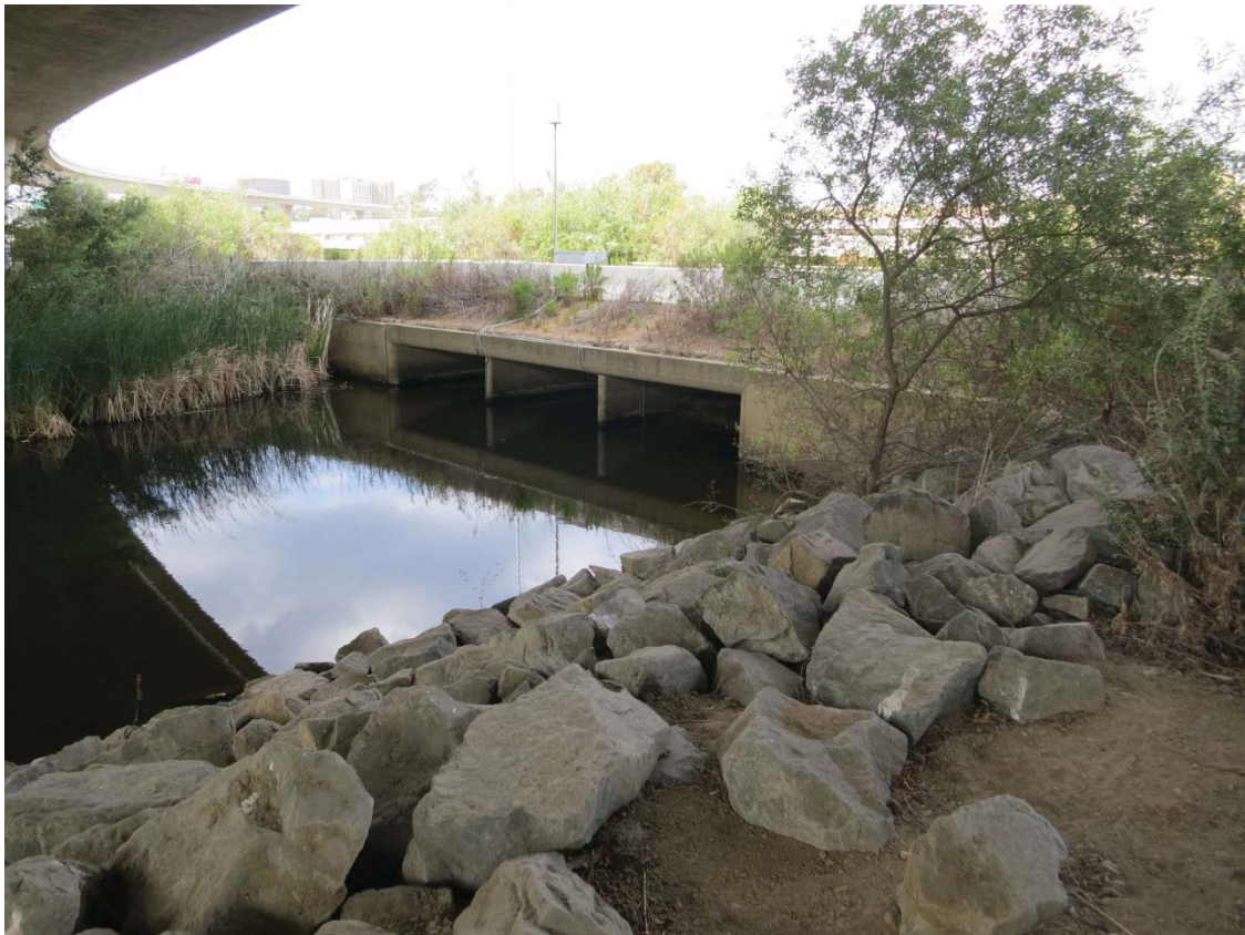
Figure 7. Box Culverts under Sorrento Valley Road at Downstream End of Reach 2
