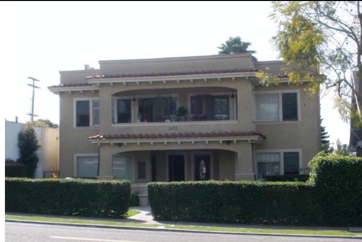
HRB #208-258 - 2473-2479 Market St (note battered porch piers)
