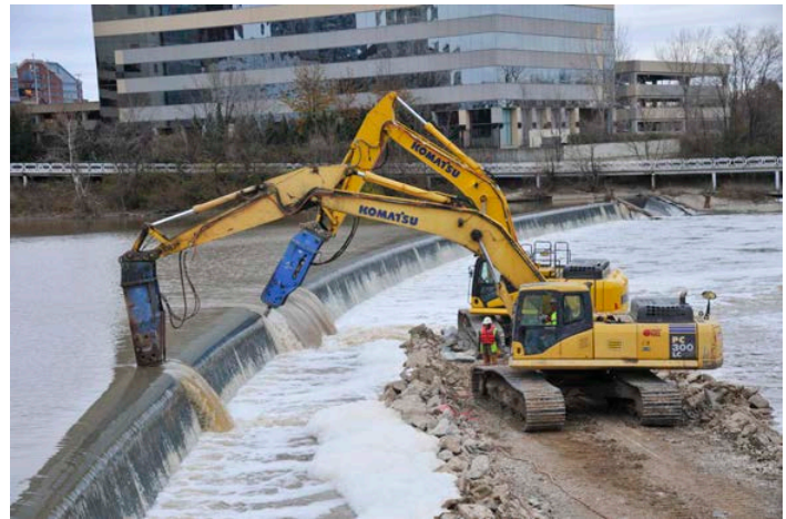
The notching of the Main Street Dam began in November of 2013 and before the start of 2014, what had been an impediment in the life of the river for more than 100 years was completely gone.
