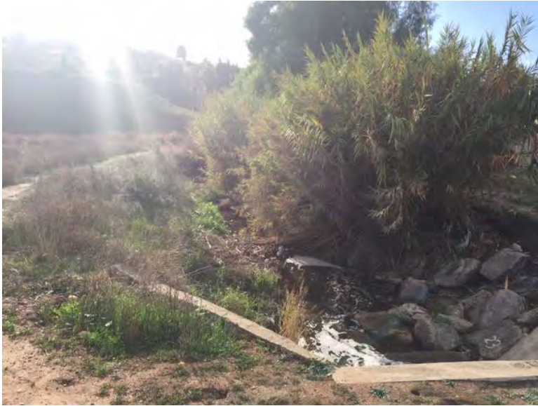
Photograph 3: Looking downstream from above the 69 th St. culvert outlet at the channel and large stands of Arundo growing up in the east end of MMP Map 115; Figure 3.
