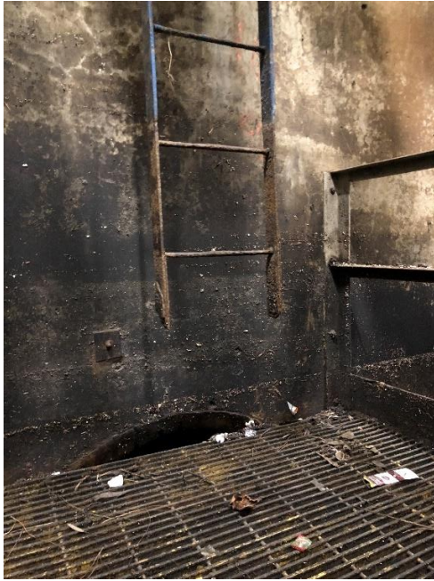
Photo taken January 13, 2023 of access ladder leading to catwalk with bottom foot of ladder missing.
