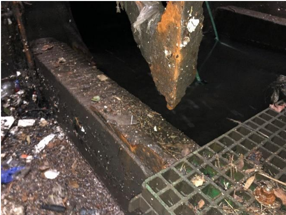
Photo taken January 13, 2023 of deteriorated catwalk support.
