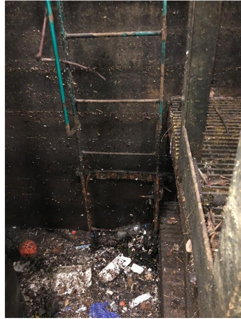
Photo taken January 13, 2023 of access ladder leading to wet well with damaged steps.
