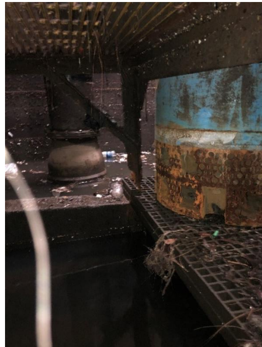
Photo taken January 13, 2023 of 2 nd location of deteriorated catwalk support.
