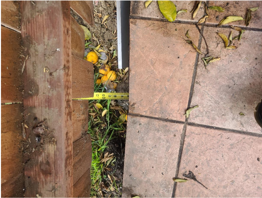
UNDERMINED WALKWAY AT 4310 EBERSOLE DRIVE
