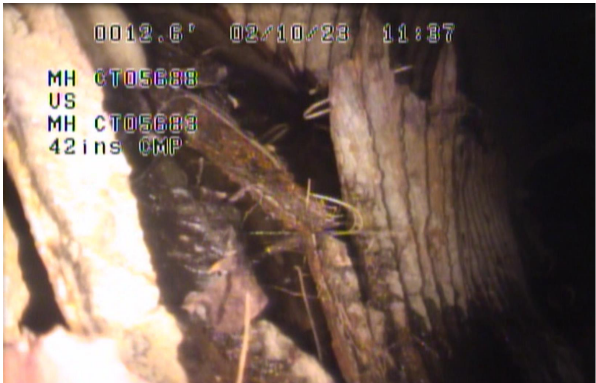
LARGE OPENING AT THE FLOWLINE
