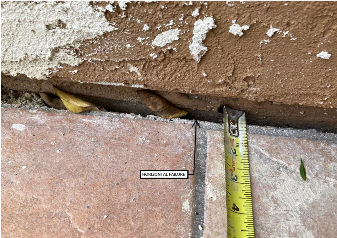
SURFACE IMPROVEMENT FAILURE AT 4310 EBERSOLE DRIVE
