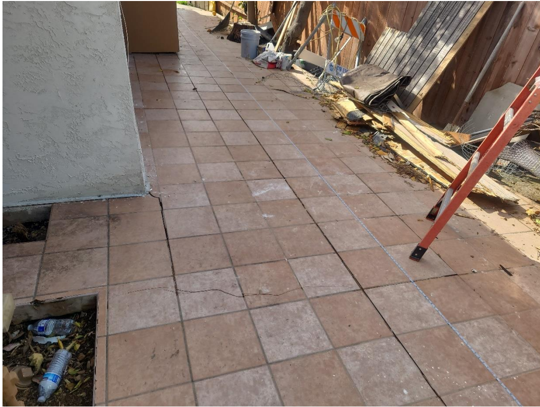
SURFACE IMPROVEMENT FAILURE AT 4310 EBERSOLE DRIVE
