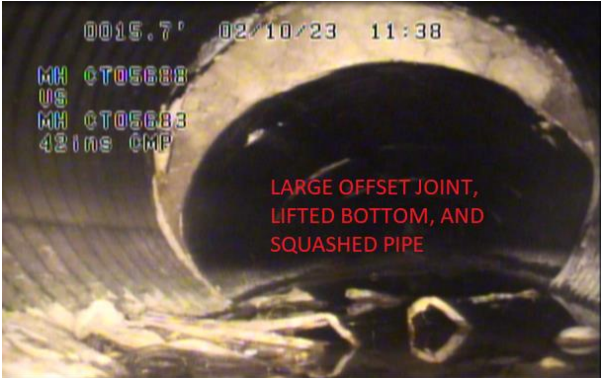
LARGE OFFSET JOINT, LIFTED BOTTOM, AND SQUASHED PIPE
