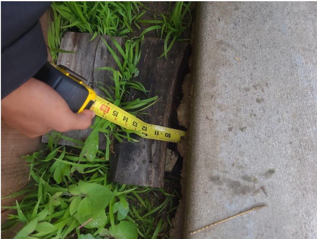
UNDERMINED WALKWAY AT 4304 EBERSOLE DRIVE
