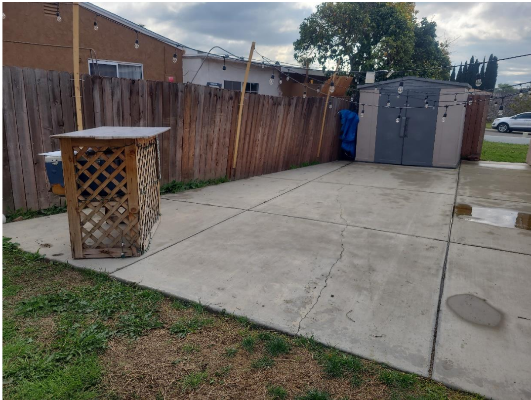
LINEAR CRACKED ON CONCRETE SLAB AT 4310 EBERSOLE DRIVE
