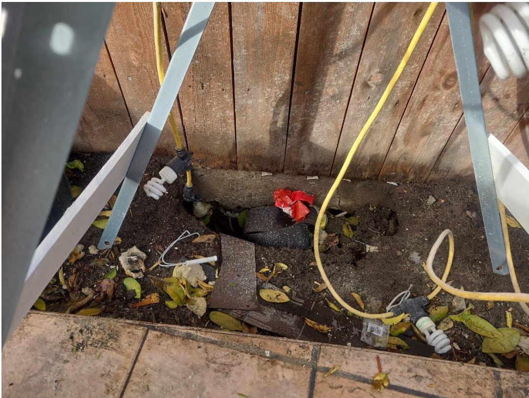
SECOND SINKHOLE AT 4310 EBERSOLE DRIVE
