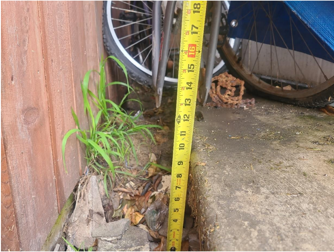
SECOND SINKHOLE AT 4304 EBERSOLE DRIVE
