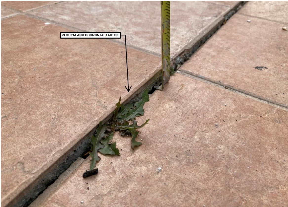
SURFACE IMPROVEMENT FAILURE AT 4310 EBERSOLE DRIVE
