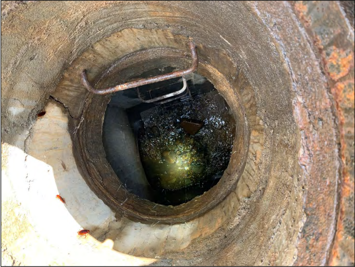
Figure 7 - Cleanout Structure Downstream filled with Debris (3/21/2023)
