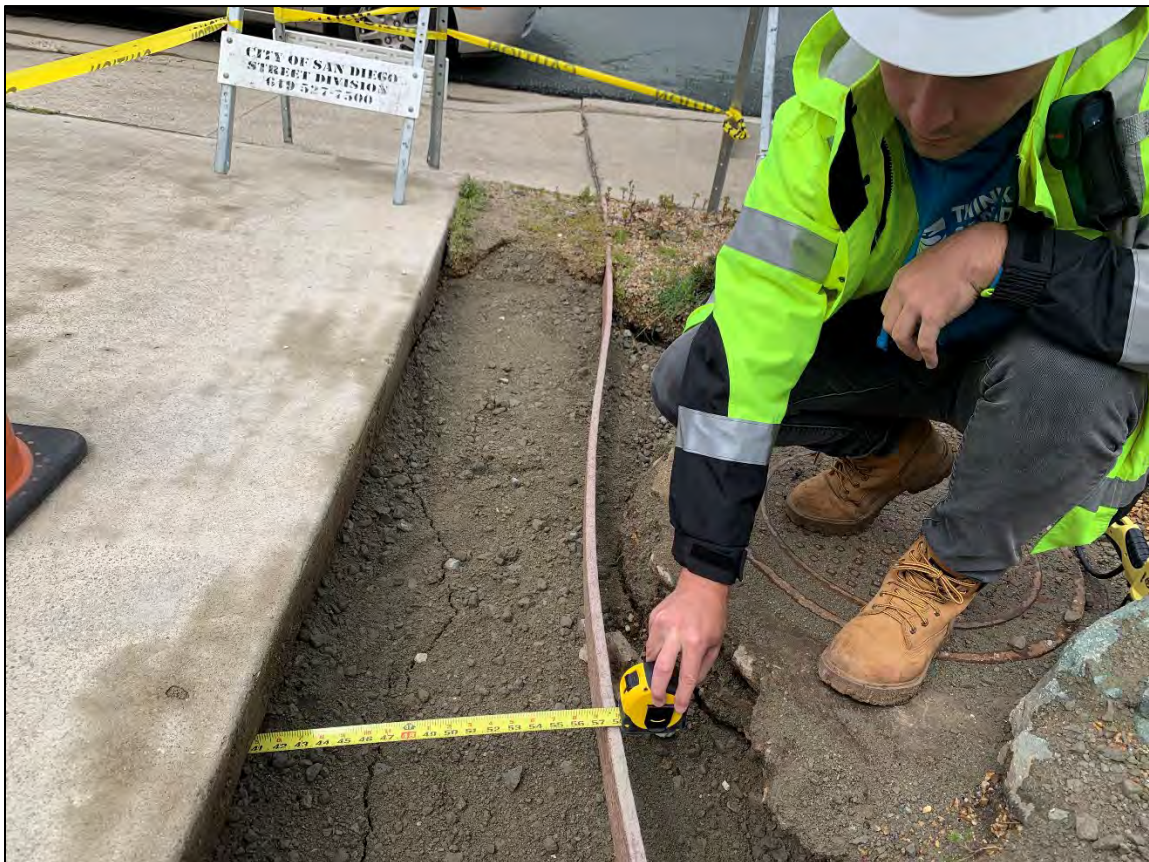
Figure 4 - Measured undermining of Concrete Slab Driveway, 42 inches (3/21/2023)
