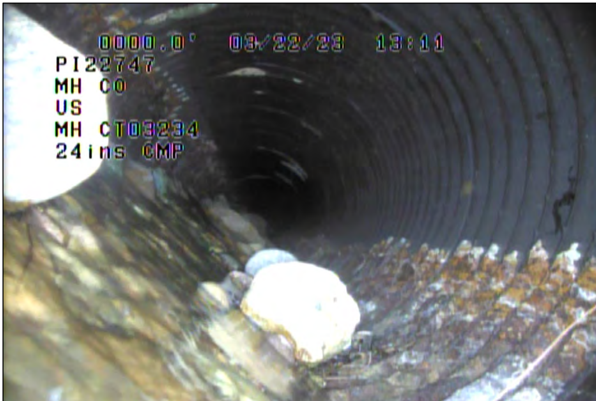
Figure 6 - CCTV of Upstream Pipe from nearest Downstream Cleanout (3/22/2023)
