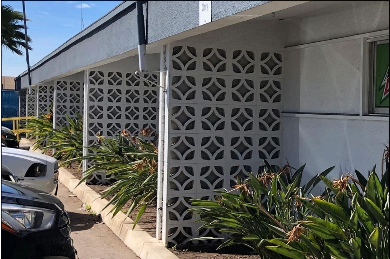
Fig. 25. Decorative pierced block screens on the Pepsi Cola bottling plant at 7995 Armour Street. IS Architecture, 2018.
