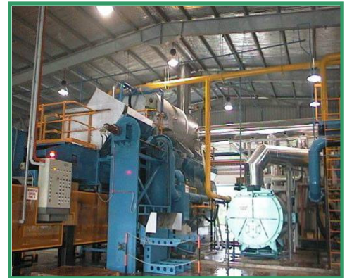
Entech Gasifier Genting, Malaysia
