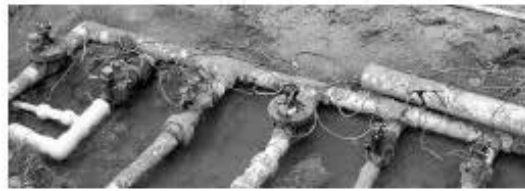
Wiring Linking Controller and Valves Source: Sueette Horspool, CC-BY-SA 3.0
