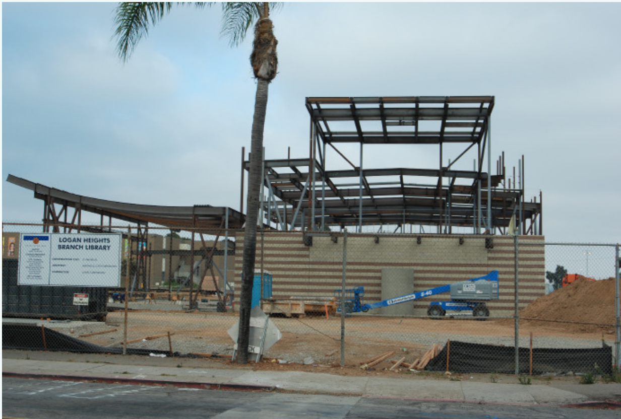
Our new library, currently underconstruction, is one place where our community will be able to access computers and internet resouces.
