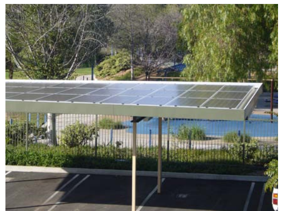
Photovoltaic panels can be mounted on roofs and carports and are a cost-effective and efficient source of renewable energy
