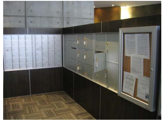
Built-in mailboxes located in an entry lobby and adjacent to signage, bulletin boards and a building directory.
