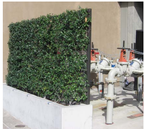
Vines are used to screen water valves and fire suppression equipment
