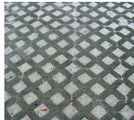
Open pavers allow water to seep into the soil, reducing potential contaminated runoff
