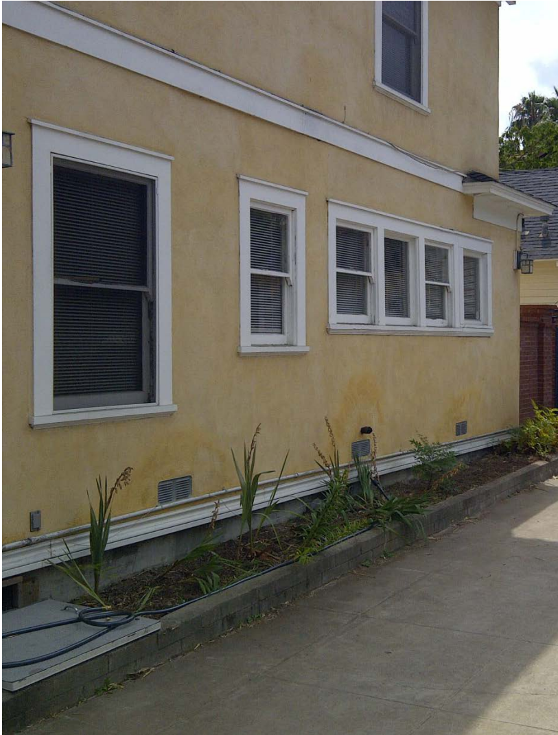
Side Windows in 2013 Prior to Unpermitted Alteration
