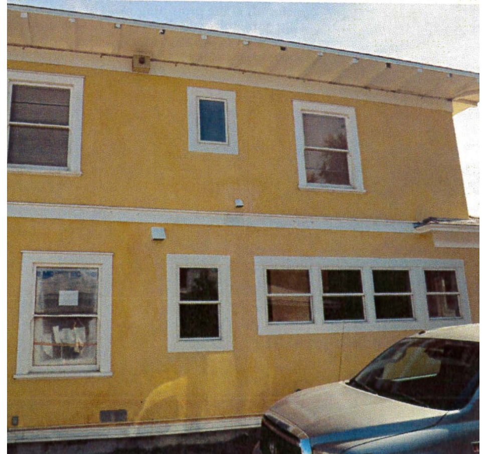
Side Windows After Unpermitted Alteration (Casing/Trim Removed, Sizes Altered)
