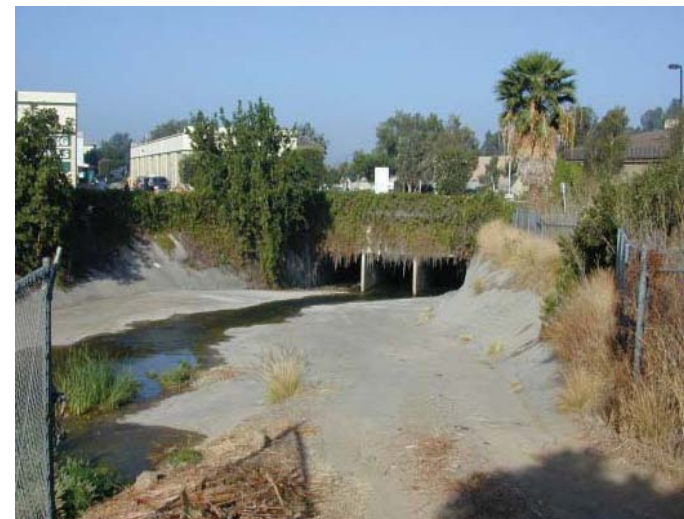
The channelization of Alvarado Creek above the Grantville Post Office offers little wildlife habitat and allows for no groundwater recharge
