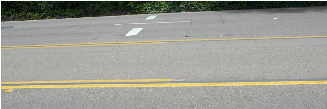
Picture 3965 - Solid Yellow and Broken Yellow Stripes on Each Side of Median
