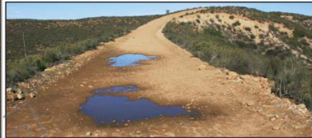
Utility road maintenance grading has created berms along the edges preventing proper drainage
