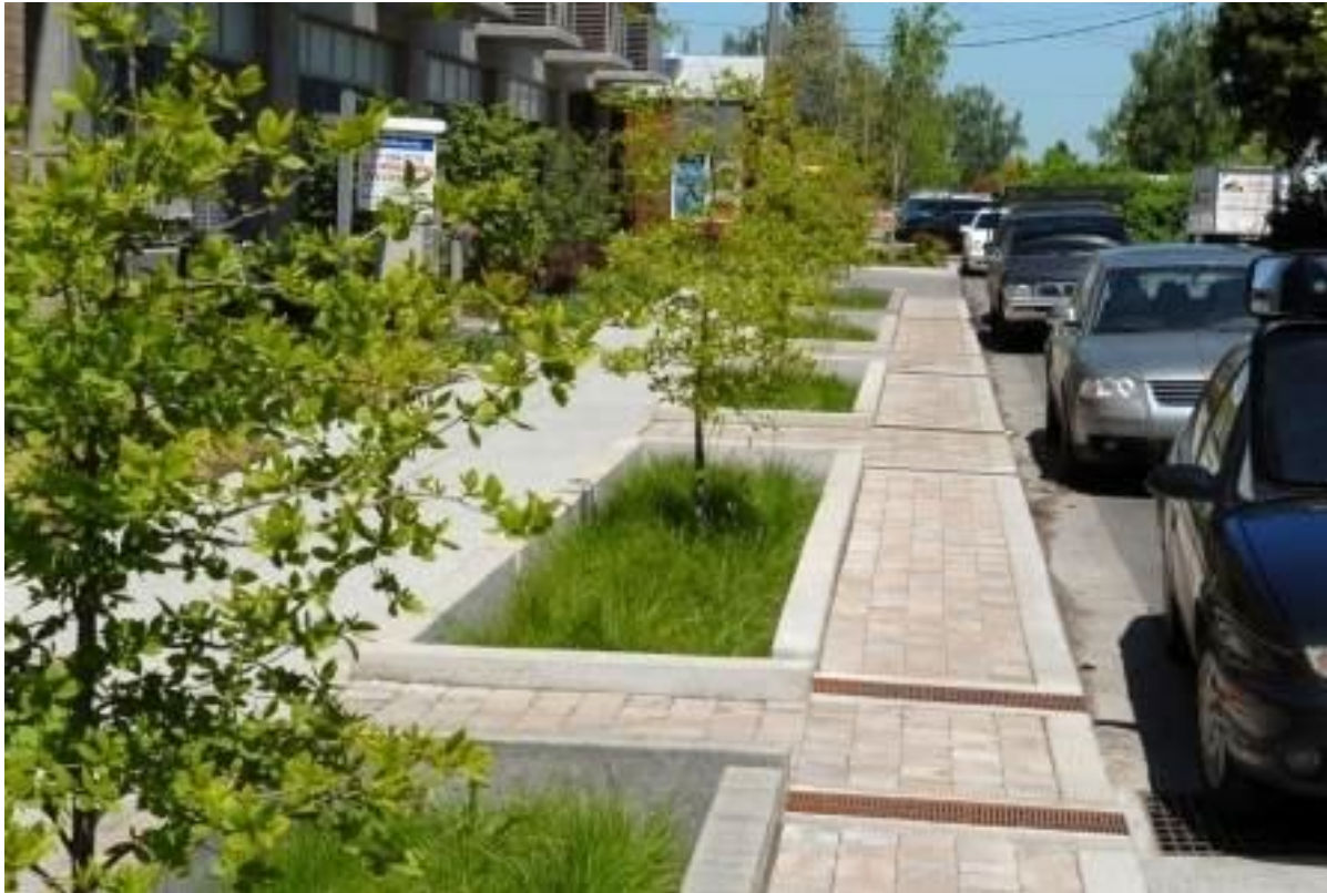
Flow-through stormwater planter
